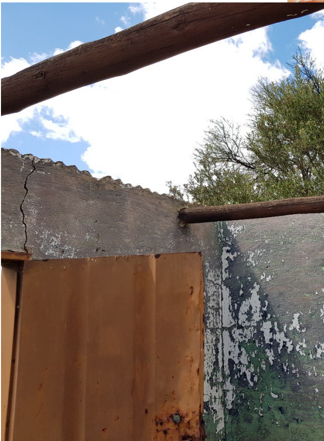
Figure 12: Indentation in cement at roof height indicate a corrugated iron roof with no ceiling. Note tarred pole rafters and custom-made doors.
