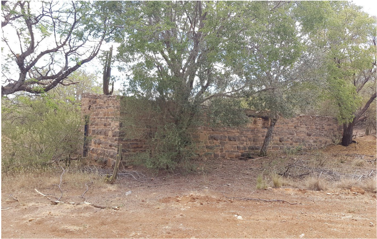
Figure 9: Back view (southern side) of barn structure with one window from the larger of the two interior spaces. The position of both front and back windows are positioned in the upper half of the walls.
