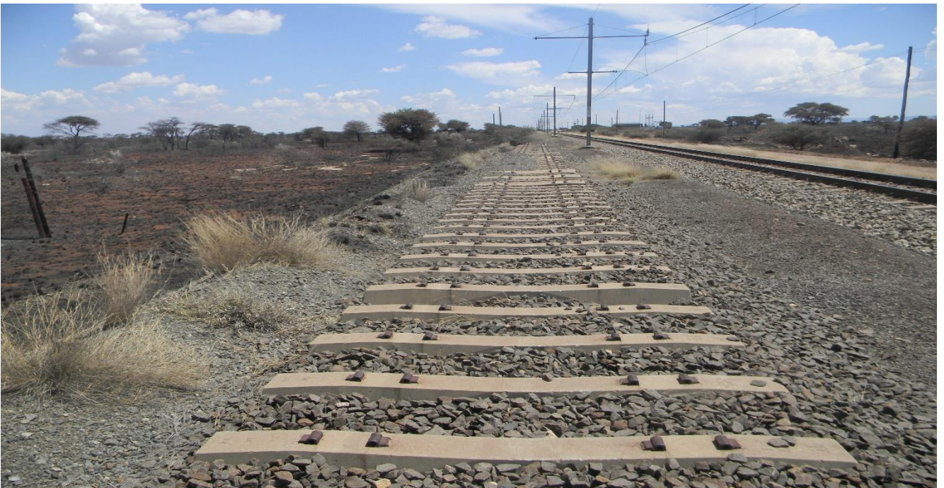
Plate 18: showing degraded sections of the proposed site.
