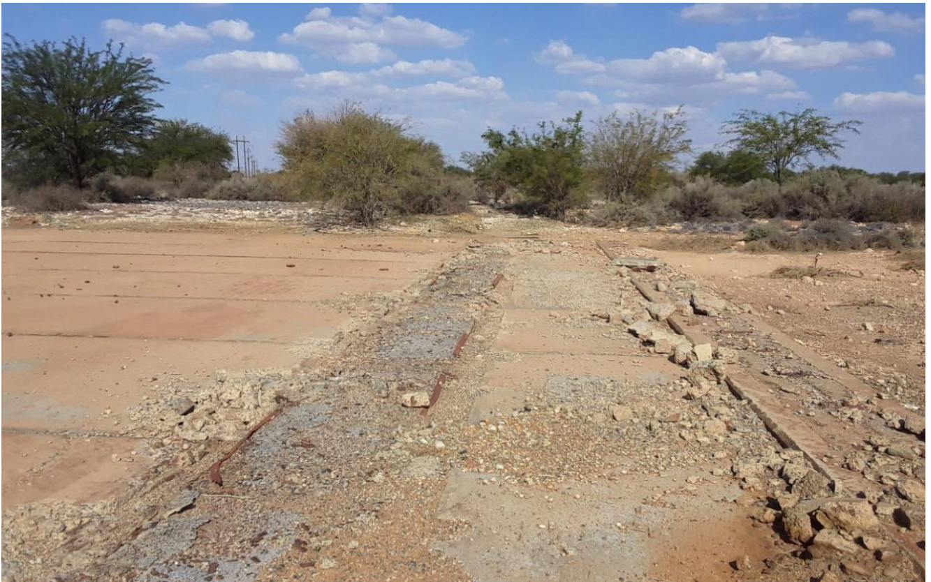
Plate 2: Photo 2: View of old demolished building 20m west of the substation (Photograph © by Author 2021).
