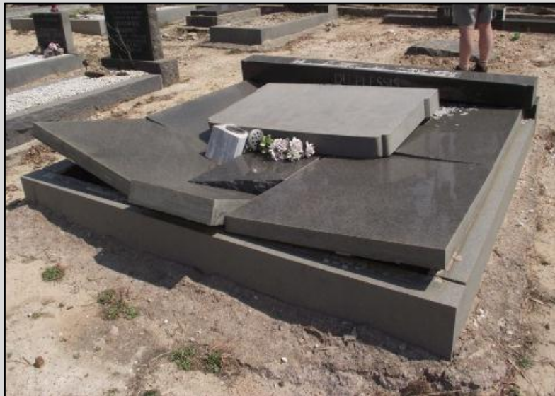
Figure 92 – Damaged slabs and headstone
