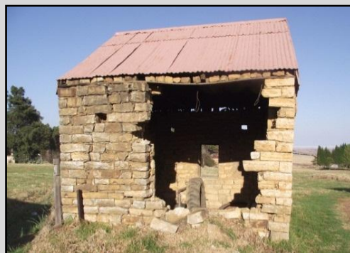
Figure 22 – PP 007: Dilapidated square structure
