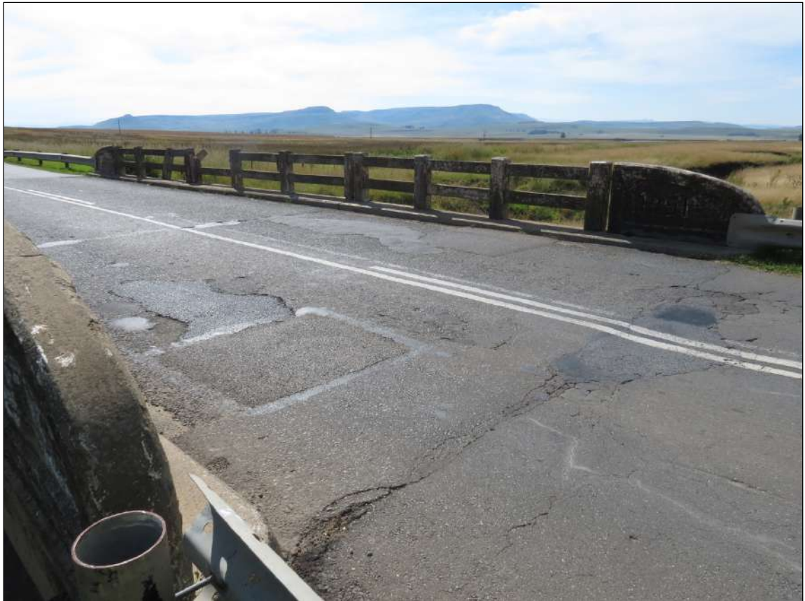
Figure 21 – Another view of the bridge at Mat 3, this view was taken in a north-western direction across the road width of the bridge.
