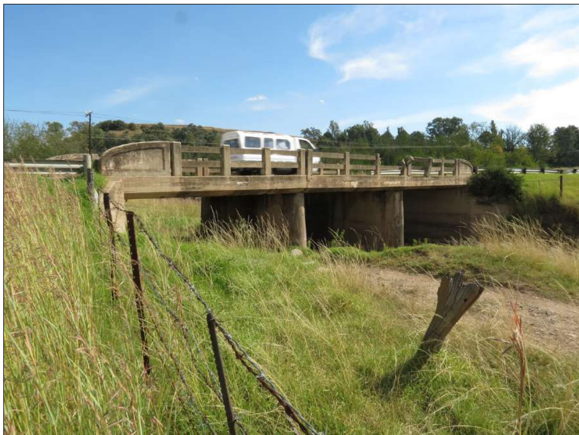
Figure 20 – General view of the concrete bridge at Mat 3 as seen from the north.
