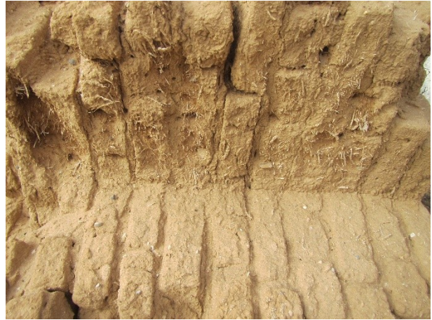
Figure 38: View of a section of fallen brick wall from the main house at De Boom 2018/002 (waypoint 002) showing locally made sundried bricks containing wheat stalks.
