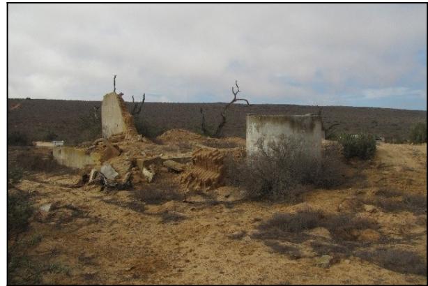
Figure 36: View of the southeast corner of the main house at De Boom 2018/002 (waypoint 002) showing the last remaining standing wall at left and a small cement reservoir towards the right.
