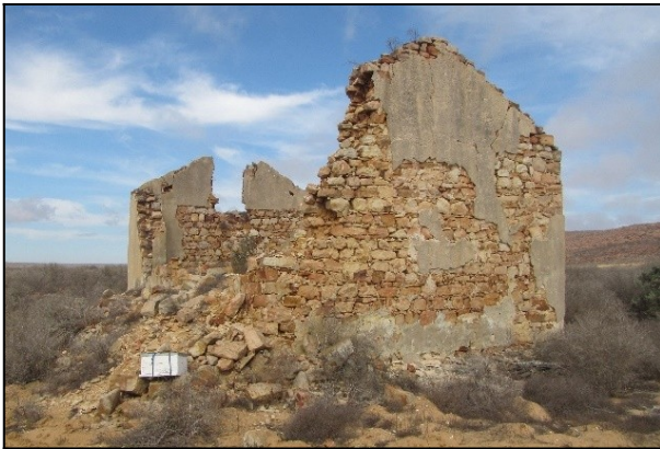
Figure 35: View of the northwest corner of the cottage ruin at De Boom 2018/002 (waypoint 002). Most walls are still standing but all joinery is absent.
