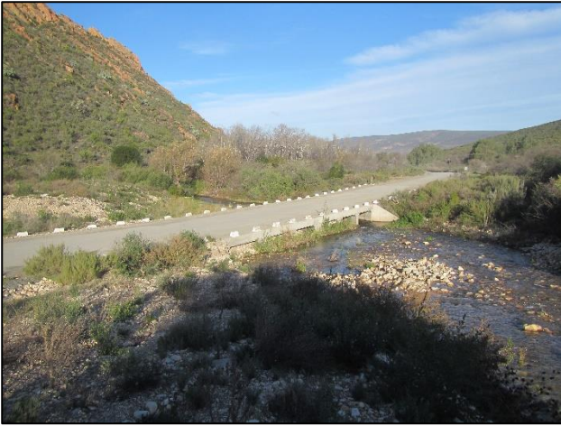
Figure 2: Current river crossing at km 57.1. Note siltation and grass growth under culvert.
