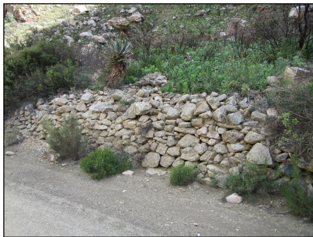
Figure 34: View of the stone retaining wall located along the road at waypoints 674-675.
