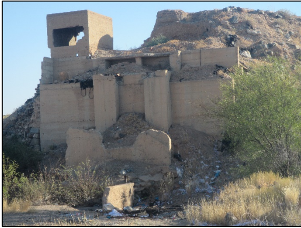
Figure 12: View of the ruined processing infrastructure located at the end of the road in Figure 4.
