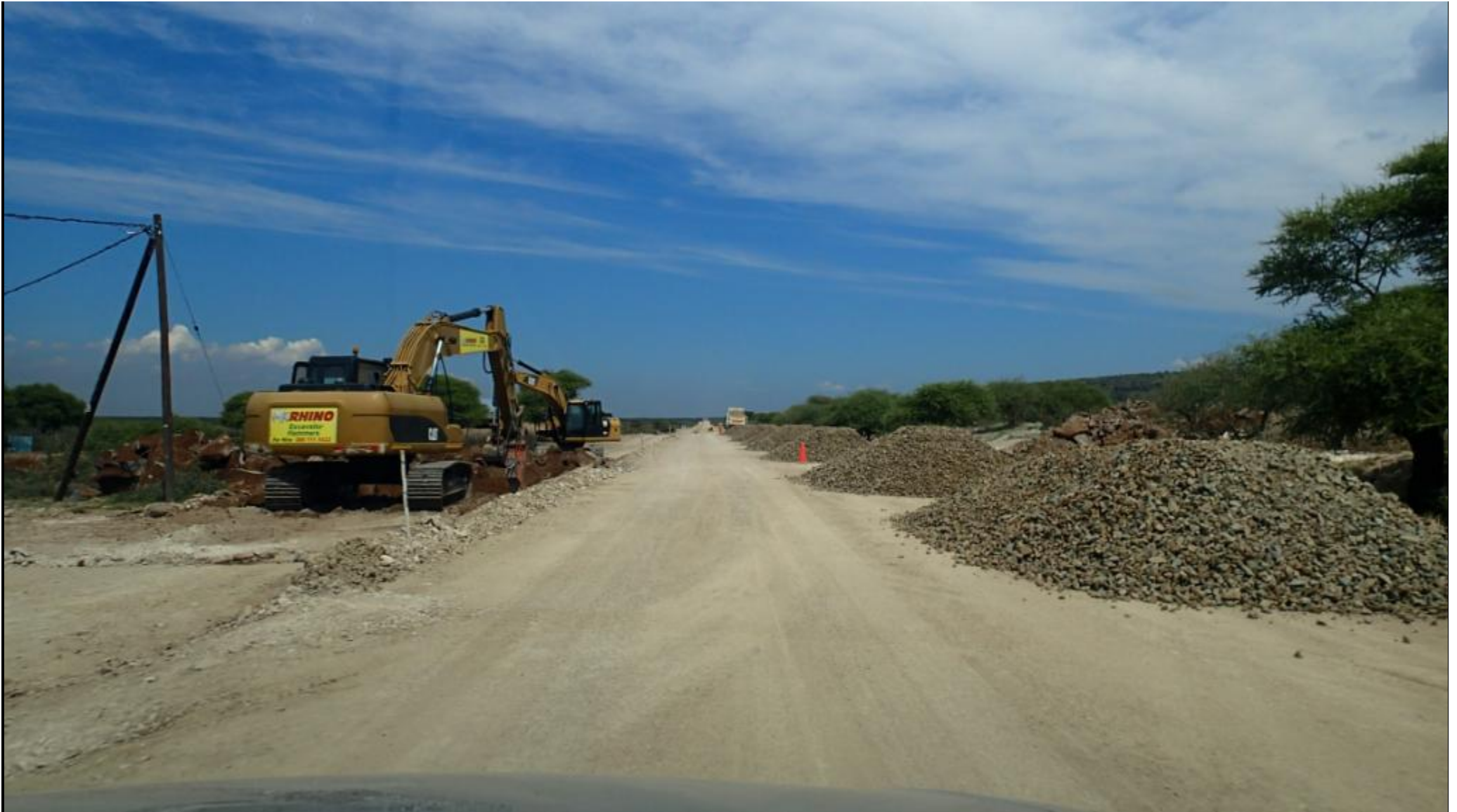
Component No. 4: Road Thomeng – Photograph of Road Construction Works between Norlim and Thomeng Village
