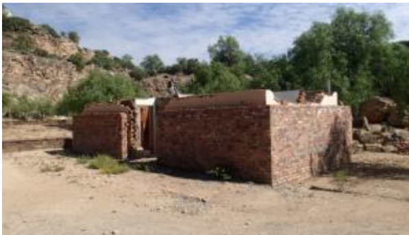
Photograph 3: Component 2 - The ablation facility at the Blue Pools picnic site is under construction.
