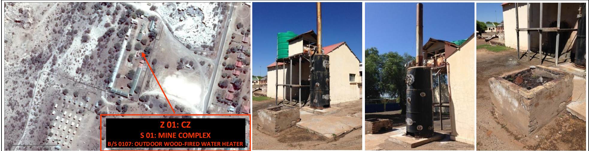
FIGURE 16 • PHOTOGRAPH 16 • Zone 01 [Z 01]: Core Zone [CZ] • Site 02 [S 02]: Mine Compound Complex • Building/Structure 0116 [B/S 0116]: Outdoor Wood-Fired Water Heater • Date: 24 February 2015
