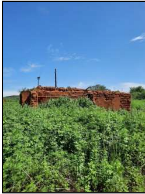
Figure 8.7. Southern view of degraded mudbrick structure at R003.
