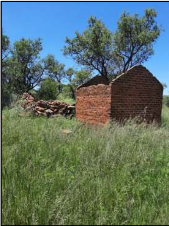
Figure 8.12. Degraded brick structure at R009
