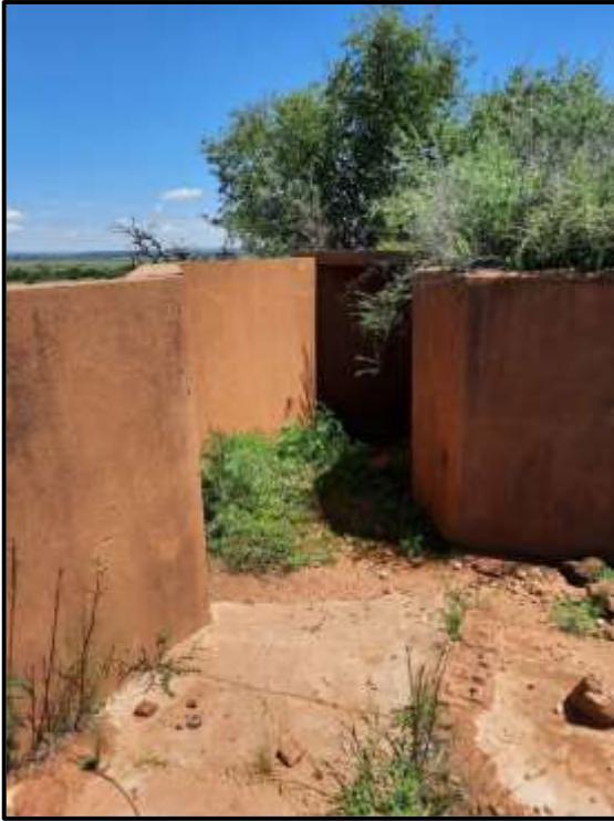
Figure 8.10. Broken down and degraded cement and brick structure at R008.
