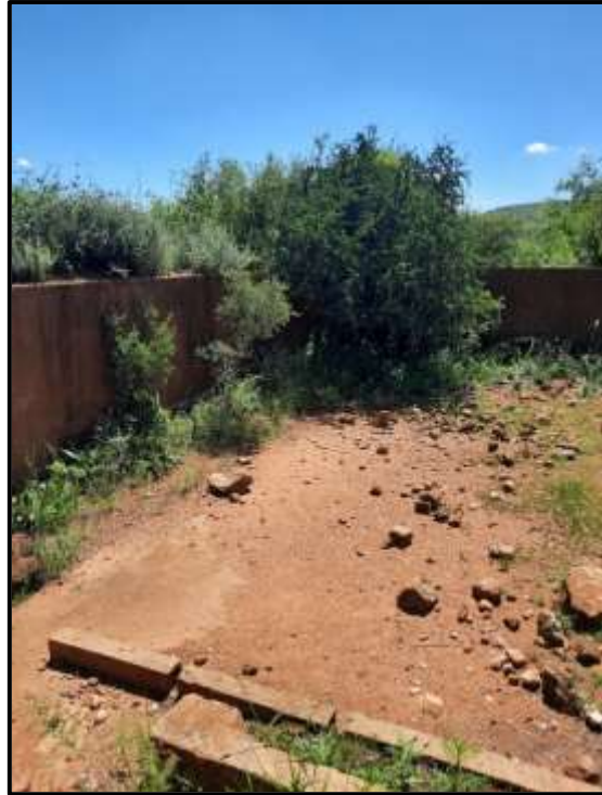
Figure 8.11. Broken down and degraded cement and brick structure at R008.
