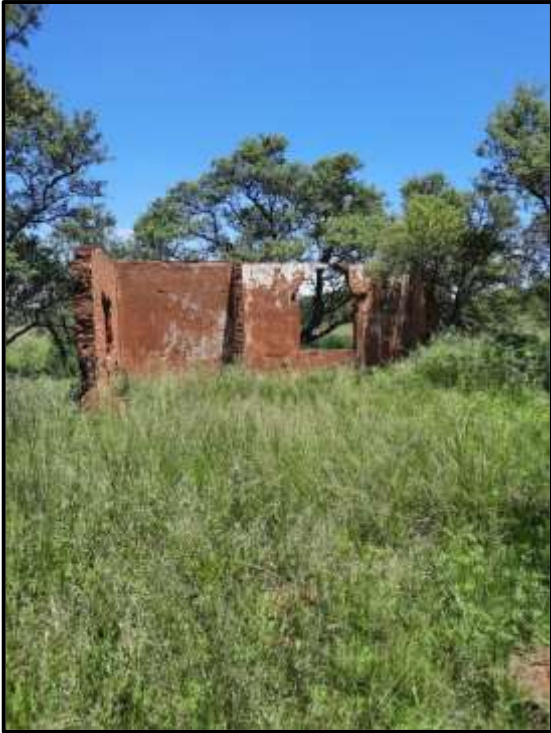
Figure 8.14. Degraded structure at R009 with later additions viewed from the south.
