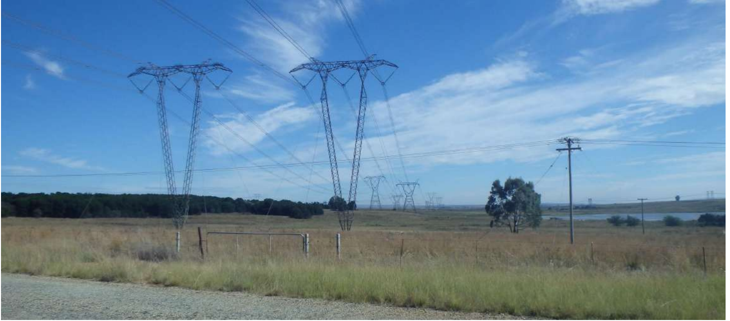
Figure 4.2: view of the large overhead powerlines crisscrossing the study area that connect to Pluto substation
