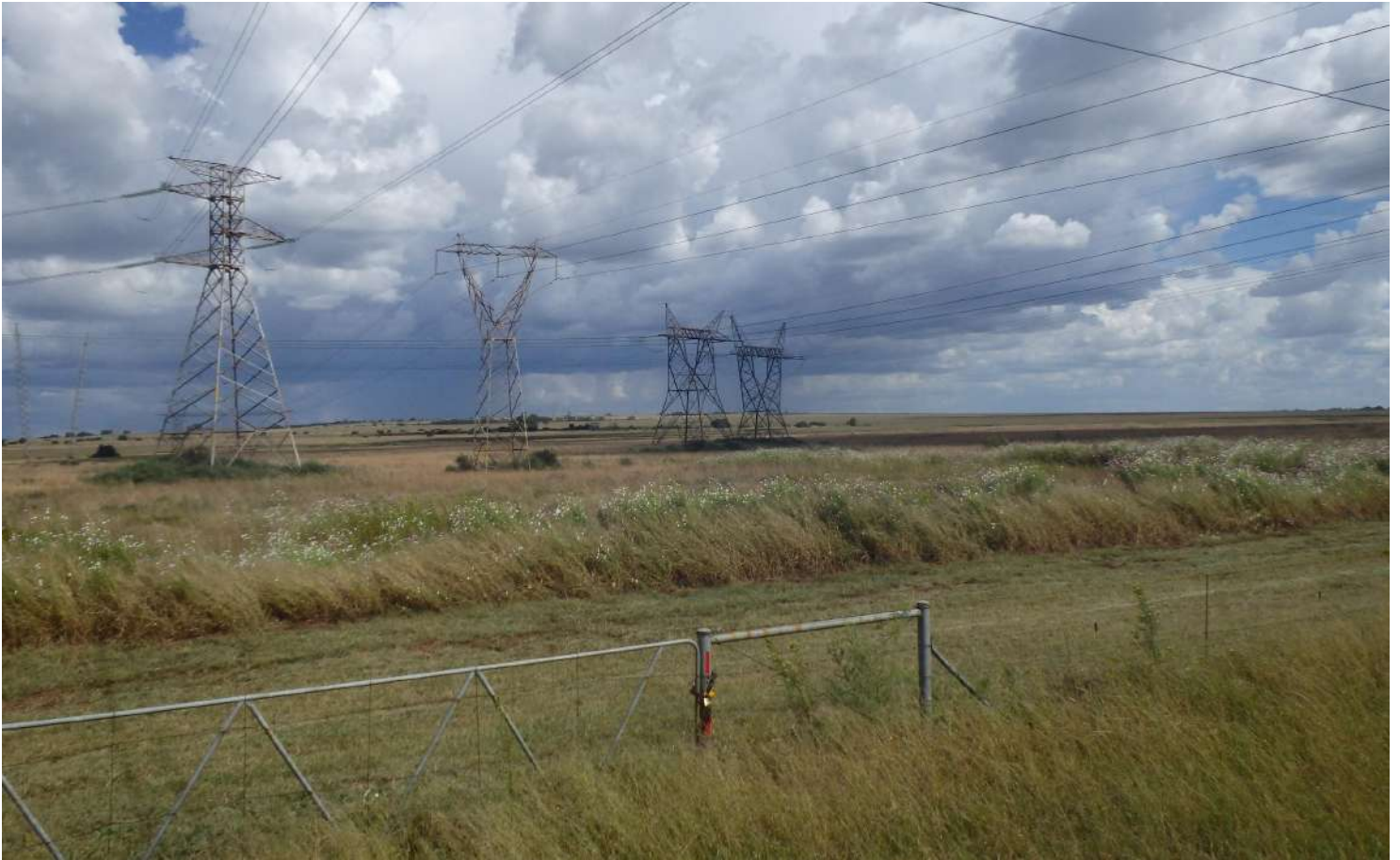
Figure 4.12: View of the connecting OHLs through Leeuwan farm
