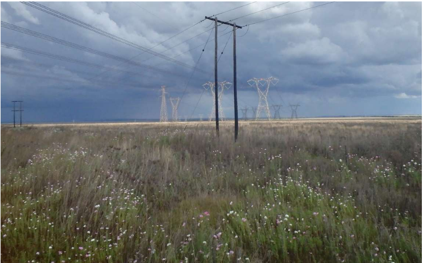
Figure 4.15: Multiple OHLs heading to the Pluto substation and onto the mining areas such as Carletonville.
