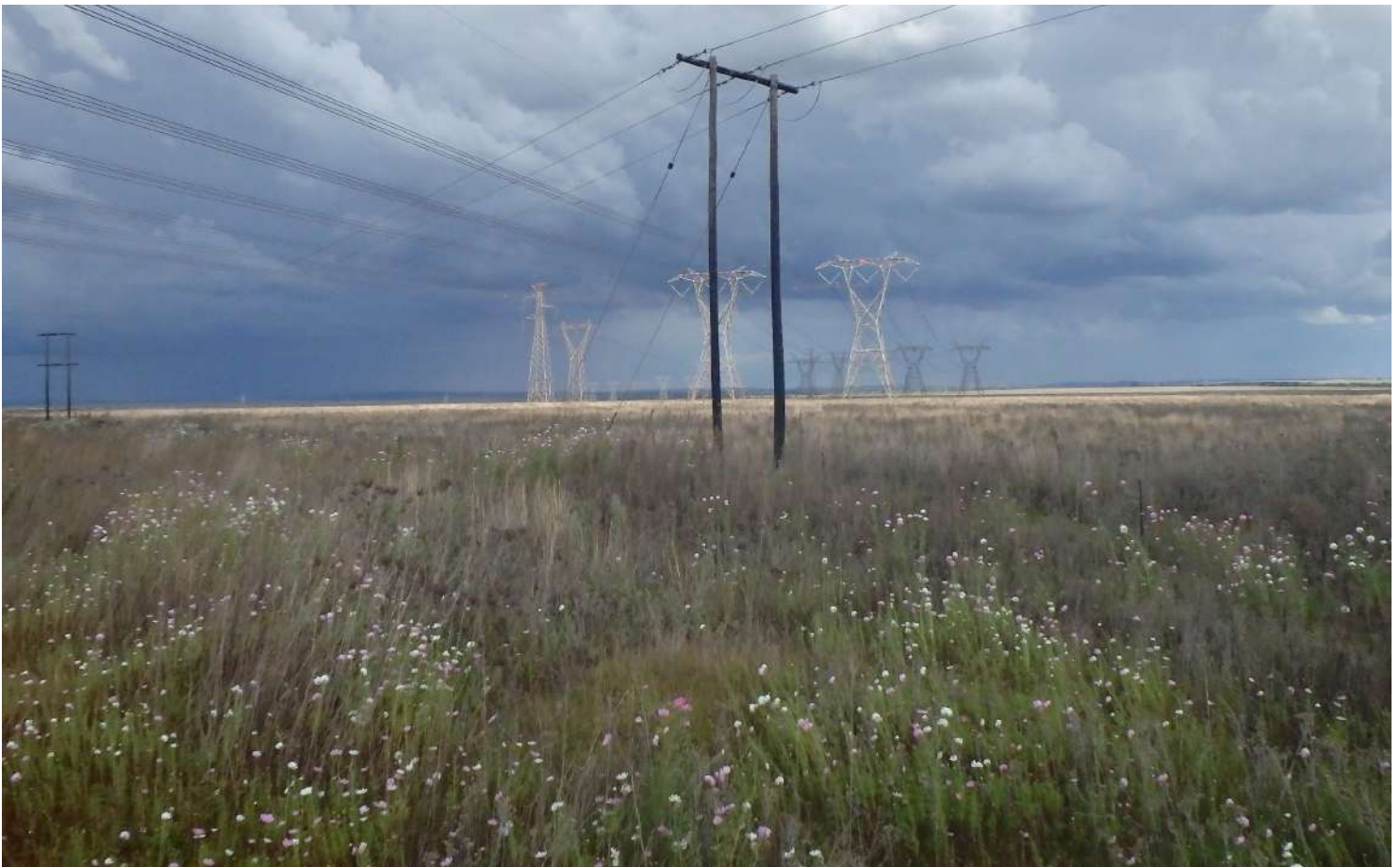
Figure 4.15: Multiple OHLs heading to the Pluto substation and onto the mining areas such as Carletonville.
