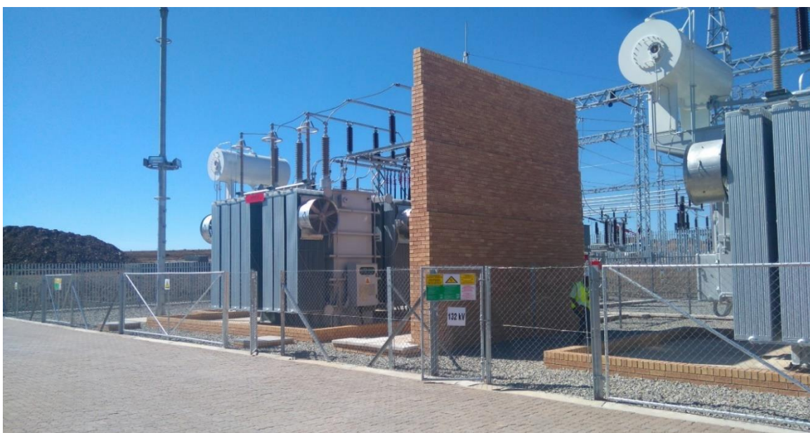
Figure 8: Example of High Voltage Transformers
