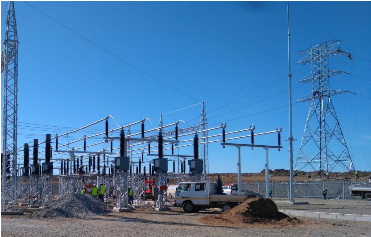
Figure 10: Example of High Voltage Transmission Line Connecting to Substation
