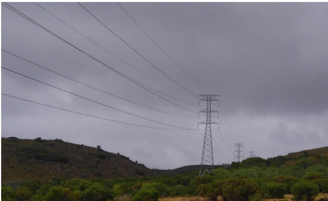
Figure 9: Example of a 132kV transmission line
