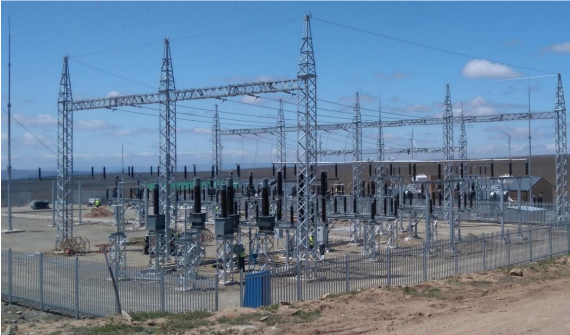
Figure 7: Example of High Voltage Substation
