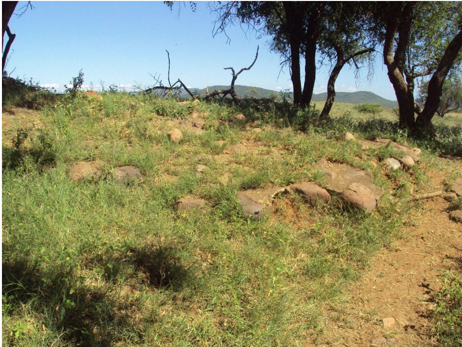
Figure 20: View of dam wall showing concentration of stones and rocks
