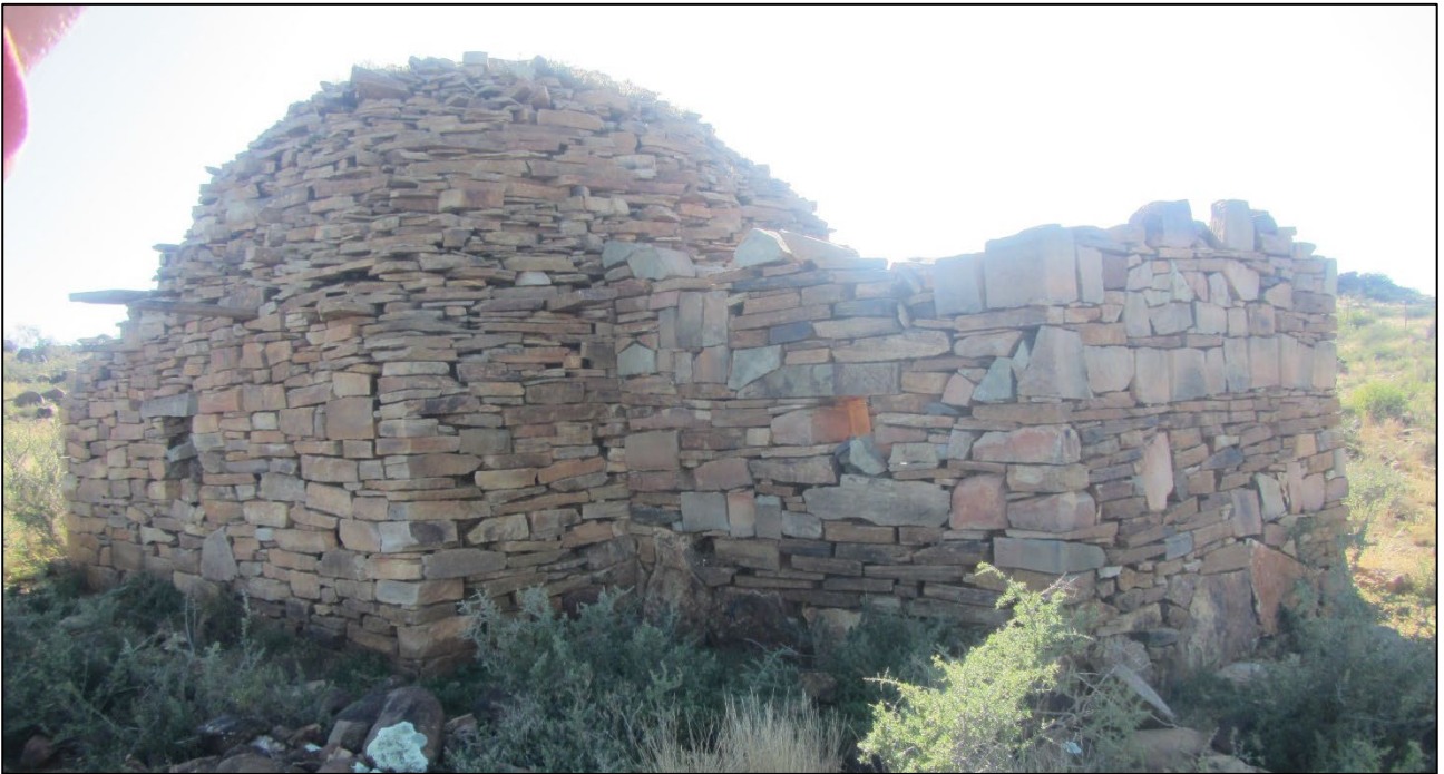
Figure 27: West and south (with added flat-roofed room) faces of the corbelled building at waypoint 1270.
