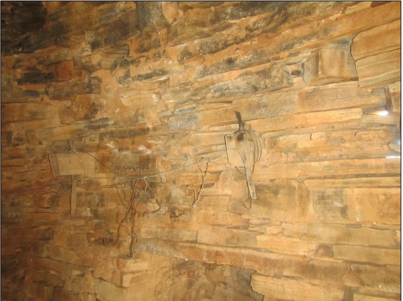
Figure 24: Internal features of the corbelled building at waypoint 1270. Two pierced wooden blocks with pegs through them are visible in the wall above the lintel of the now closed up northern door. Some wire has been fastened to the wooden blocks.
