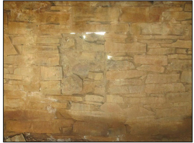
Figure 23: Closed up window in the west wall of the corbelled building at waypoint 1270.
