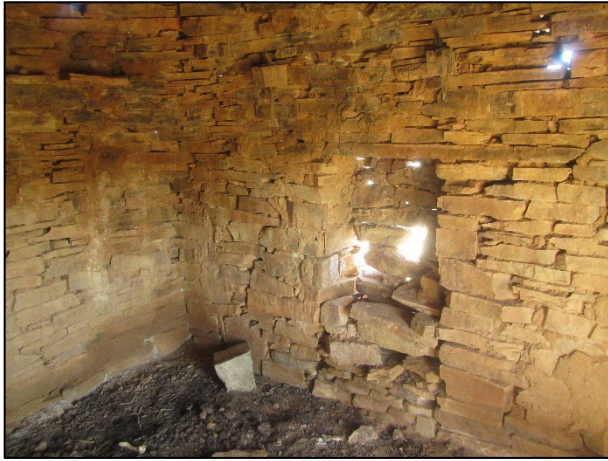
Figure 22: Closed up door in the north wall of the corbelled building at waypoint 1270.
