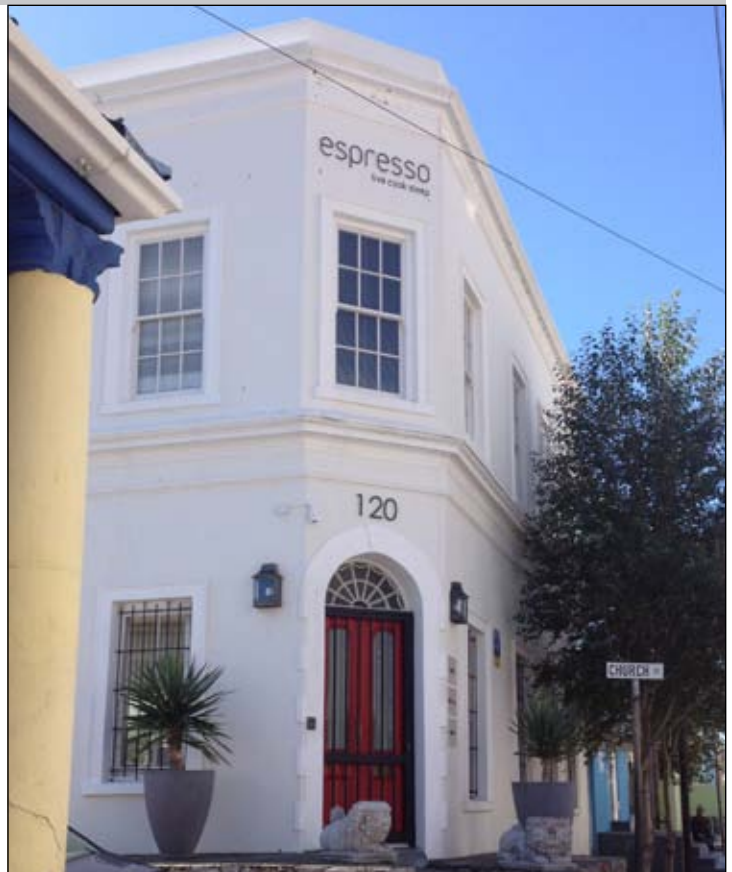
Figure 8: Timber sash windows, Georgian style garlanded, spoked fanlight and plaster mouldings are all in good condition.
