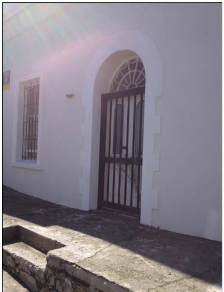
Figure 9: The secondary entrance door off Church Street indicative of the site before it was consolidated.
