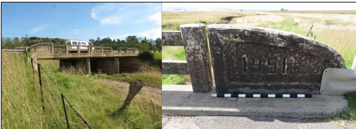
Figure 5: General view of the bridge at MAT 3 at the time of the PGS HIA study.
