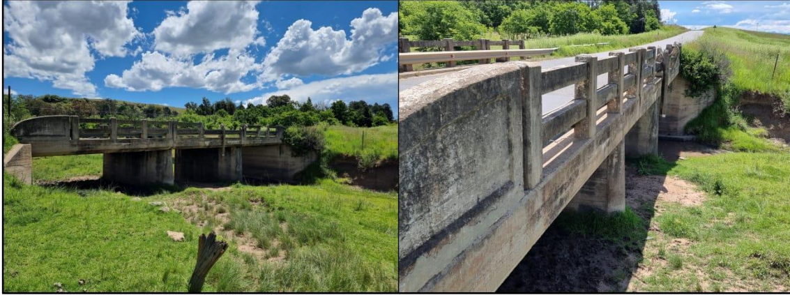
Figure 6: General view of the bridge at MAT 3 at the time of the site survey for this Memorandum
