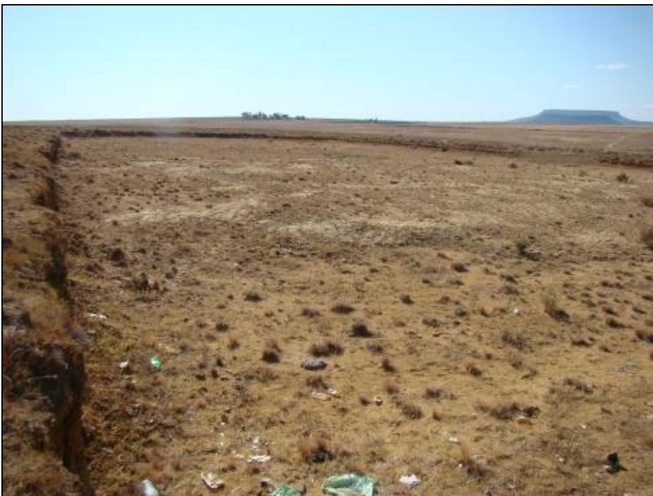
Fig.25 Trenches prepared for the burial of refuse at the new landfill site, Senekal.
