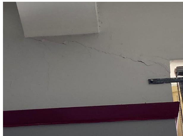
Typical crack around windows.
