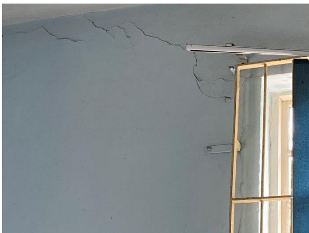
Typical crack around windows.
