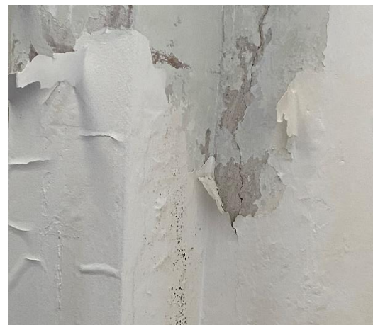
Crack adjacent to internal beam, further investigation required.
