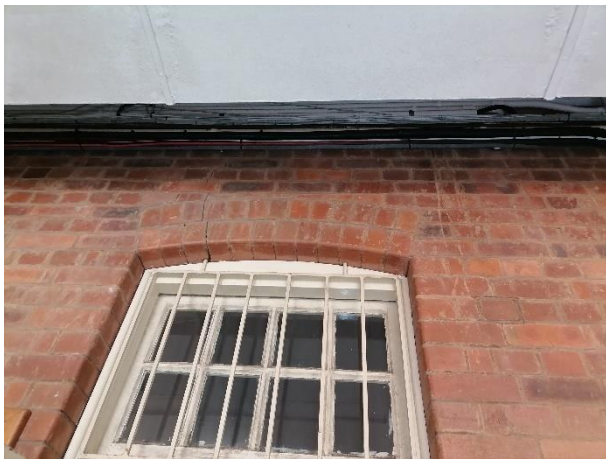
Crack on above window.
