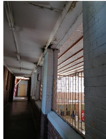
Passage : Ceiling damp and deteriorated.
