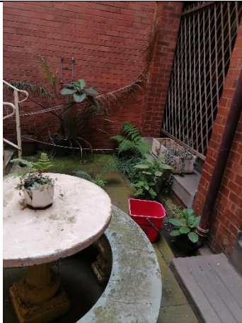
Open Courtyard: vegetation, mildew and moss.
