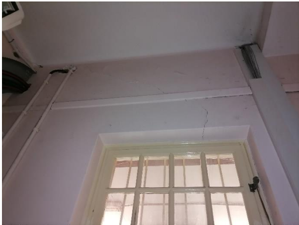
Crack on external wall coincides with internal cracks.
