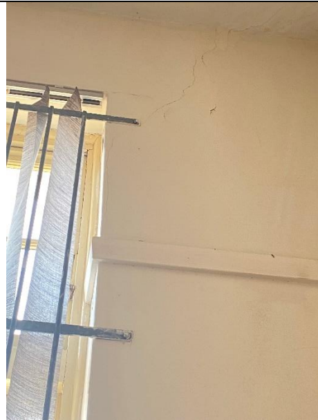
Crack on external wall coincides with internal cracks.
