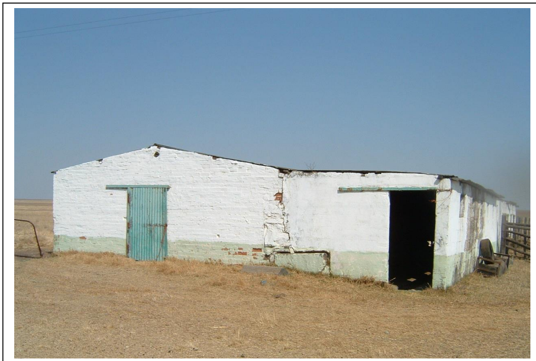
Figure 10 - A shed with a lean-to is part of FC07 which also incorporates a residence which was also constructed with bricks and cement (above).
