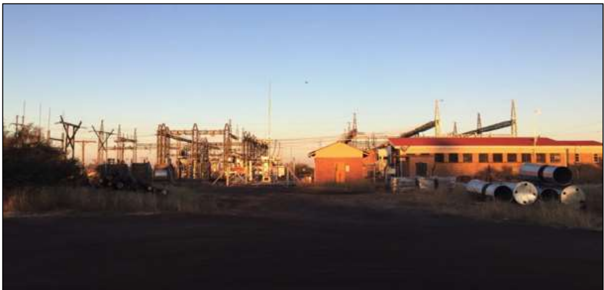
Figure 24: View west from Photo 6 of the existing Eskom Hotazel Substation to which the proposed power line would be routed.
