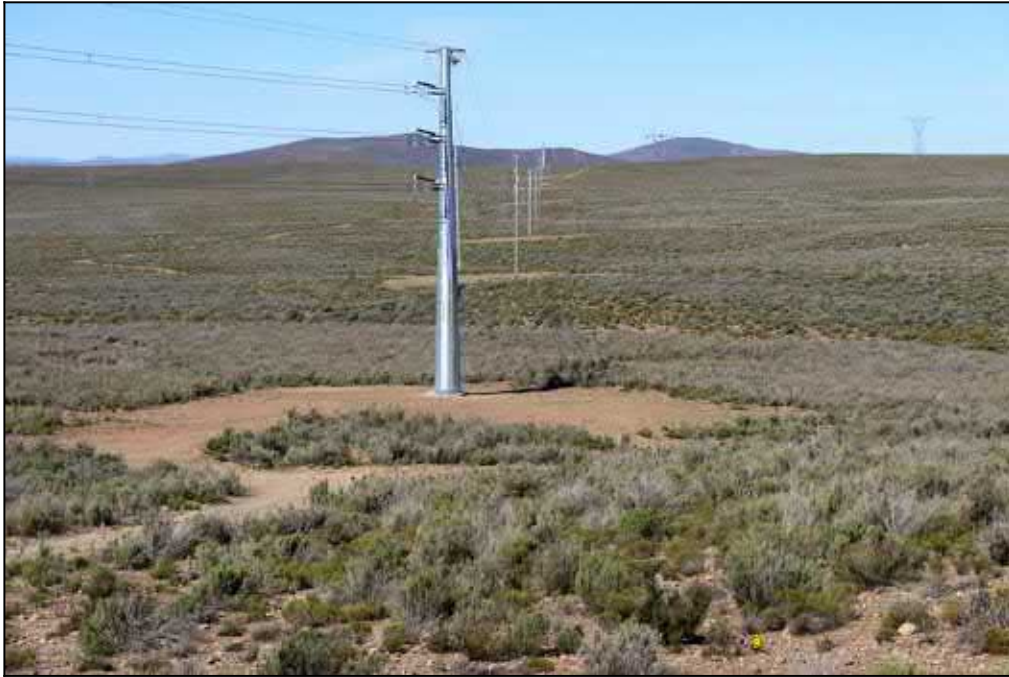
Figure 10: View eastwards along the recently constructed powerline between the new substation on Bon Espirance 73 and the Komsberg MTS. Bedrock exposure in the low relief terrain here is very limited. Any palaeontological impacts are more likely to be attributable to surface clearance than to excavations for electrical pylon footings.
