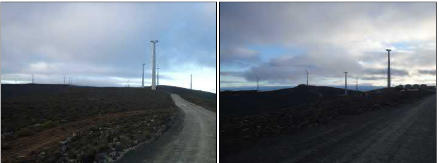
Figure 4.6: Contextual Images taken from the alignment running north-west to south-east indicating turbines under construction
