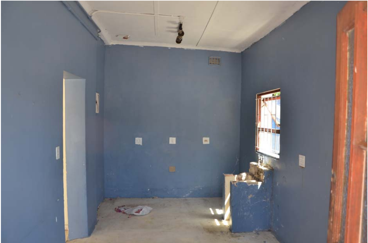
Room 8 (to be partially demolished) shows no traces of its age or time
