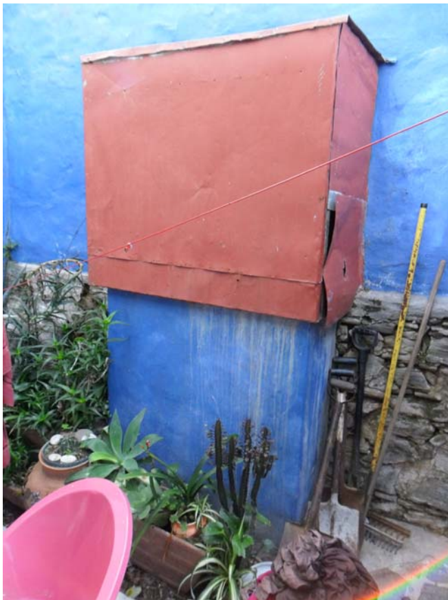
The packed stone wall that will be revealed after the proposed demolition
