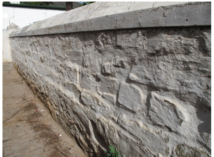
The last remaining portion of the original site boundary wall, to be demolished for the new driveway axis.
