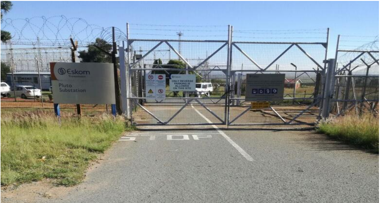
Plate 1: Photo 1: View of Pluto Substation in Gauteng where the proposed powerline will start (Photograph © by Author 2018).
