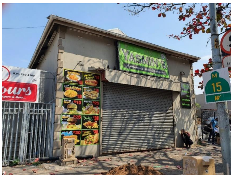
The original veranda has been bricked in, quoining added and the recessed entrance replaced with a roller shutter door.
