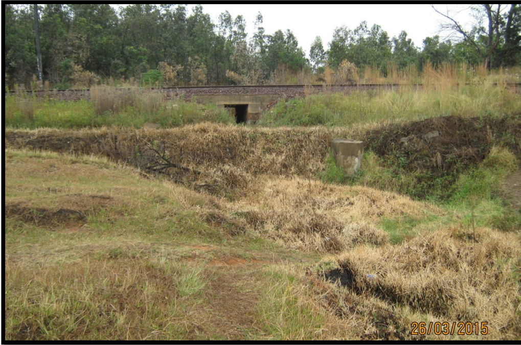
Figure 12: Northernmost corner of the development. A 1,2 km; 1,3 km; and 270 m extended stormwater trench is located on this northern border.
