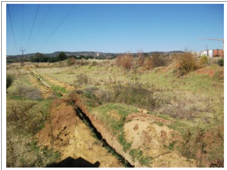
Figure 7- Disturbances and alterations along the proposed pipeline corridor include illegal mining activities by zama zamas in order to remove underground cables (above).
