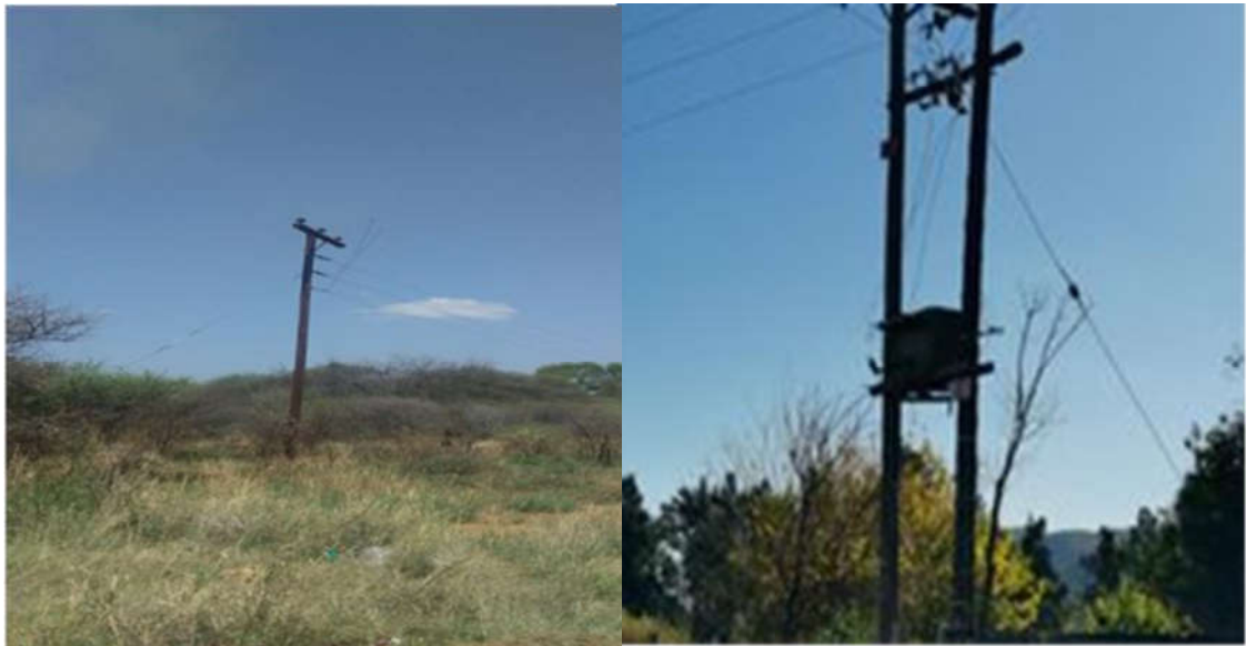
Figure 1 Existing MV Feeder line and Transformer
