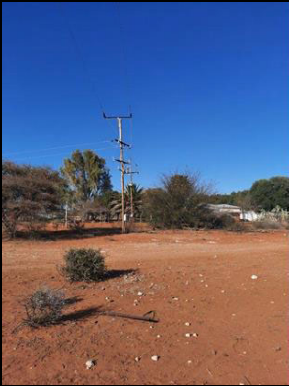
Figure 7.1. Existing Powerline infrastructure.
