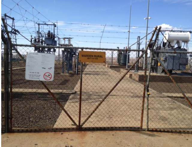
Photo#1: Warden-Rural Substation
