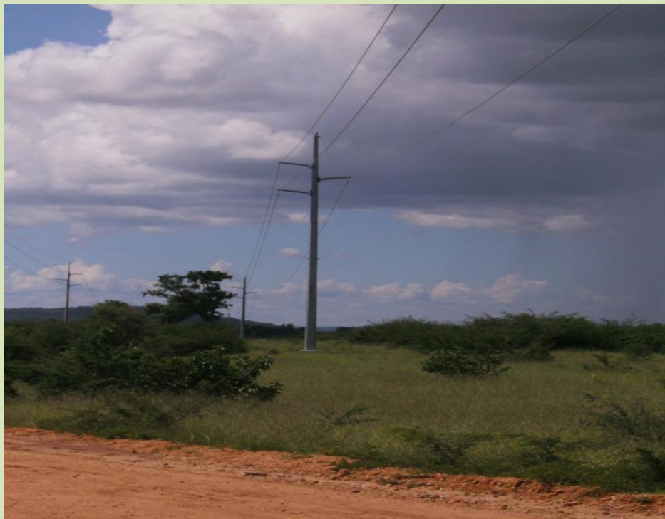
Typical Monopole Power Structure
