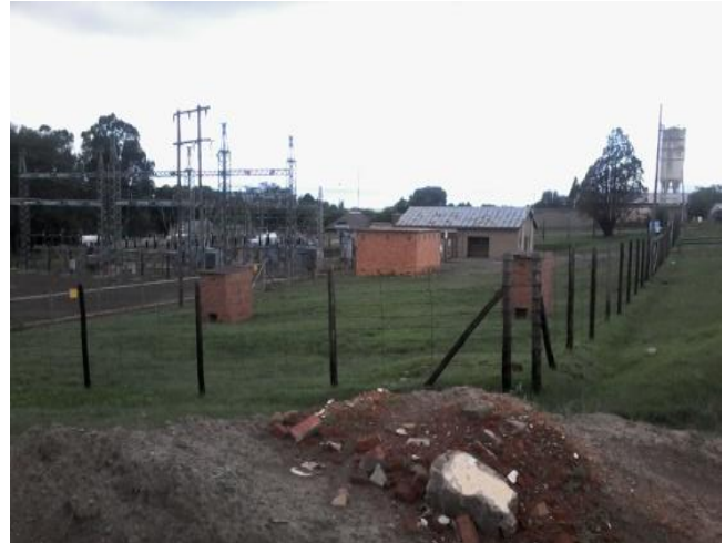
Photo#2: Vrede Municipal Substation
