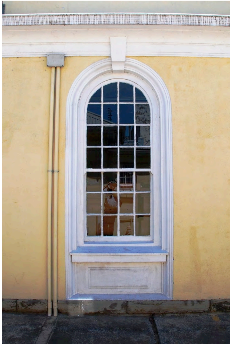
Timber sliding sash window with arched top and keystone with later surface mounted electrical conduits on lhs.
