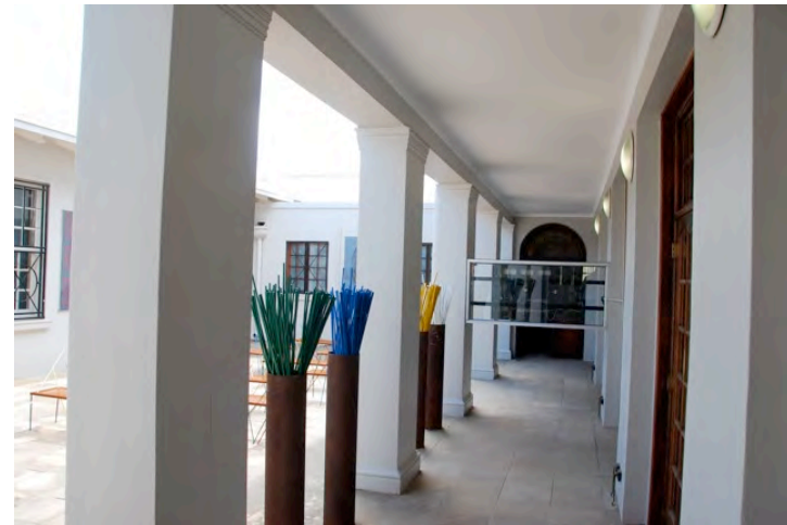
Verandah on south side of Council Chamber with modern TV monitor blocking circulation
