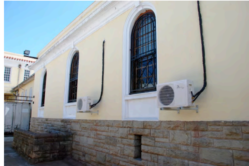
Installation of inappropriate Air-conditioning machinery
