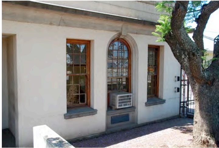
Arched window with 'keystone' flanked by sliding sash windows and insertion of air-conditioning unit.
