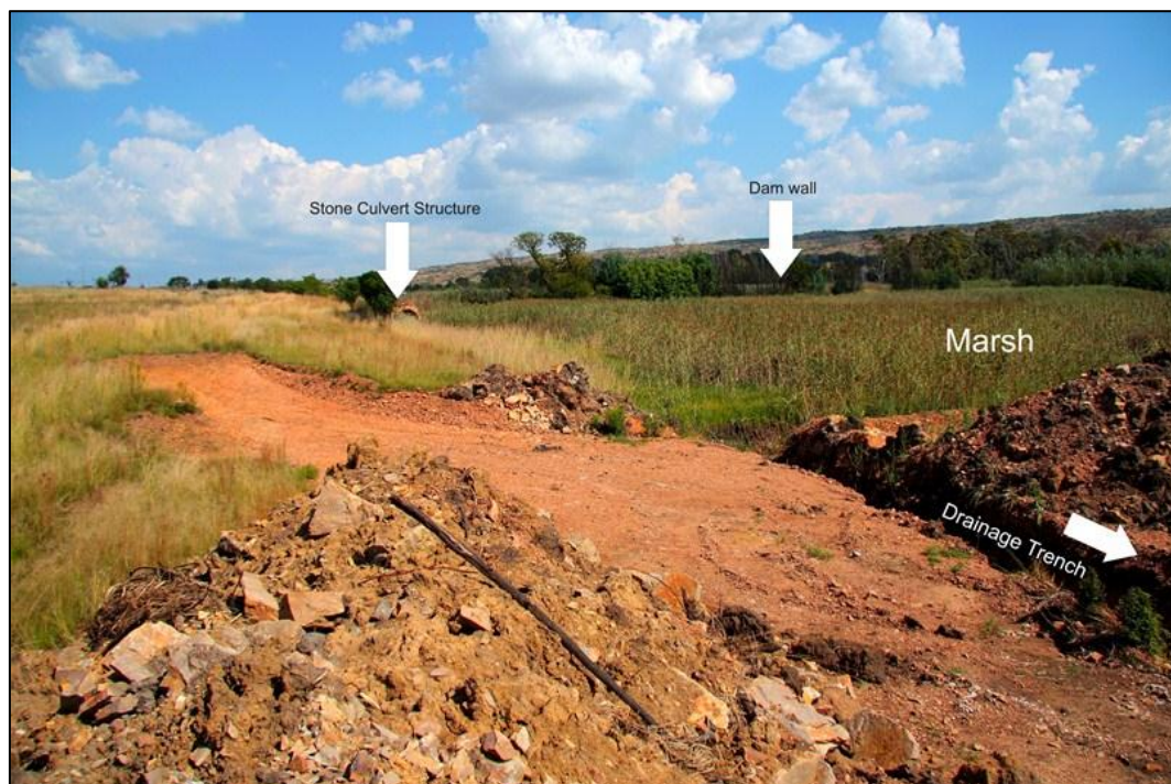
Figure 10: Position of the historical stone culvert on the southern extremity of the survey area.
