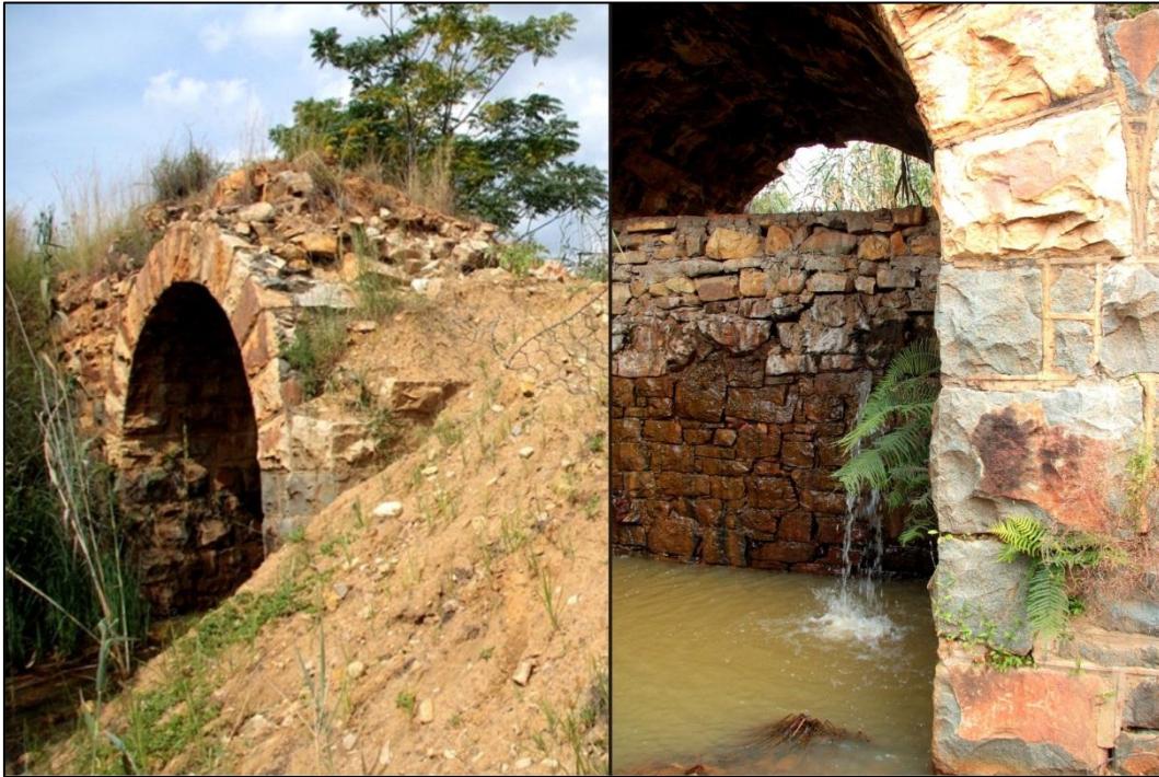
Figure 11: Partially intact historical sandstone culvert structure which currently forms part of a retaining dam wall.
