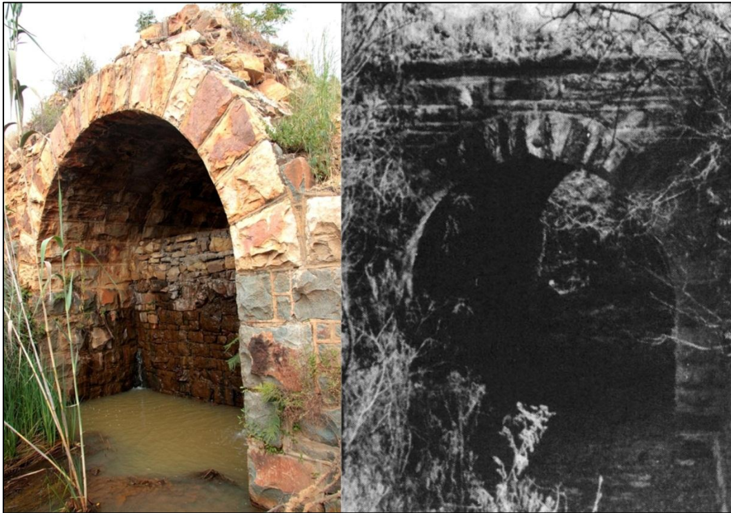
Figure 19: A NZASM culvert at Pienaarspoort (left) and another in Pretoria at the Fountains Valley (right) (after De Jongh 1988).
