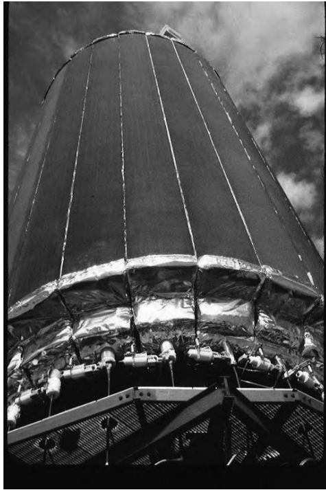
Figure 5- Receiver heat exchange panels – image courtesy NREL
