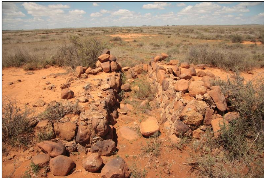
Figure 5-13: Site HO02: Dilapidated Historical Period dam wall channel.
