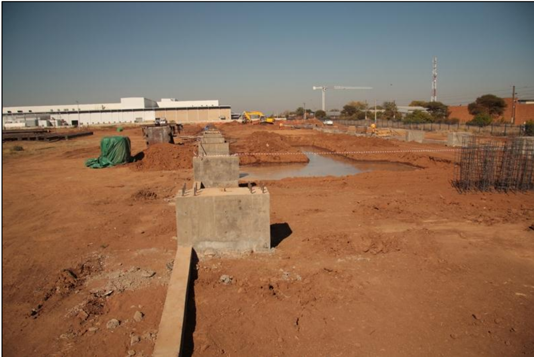
Figure 5: Infrastructure construction of the Babelegi steel recycling facility along the western sector of the property.
