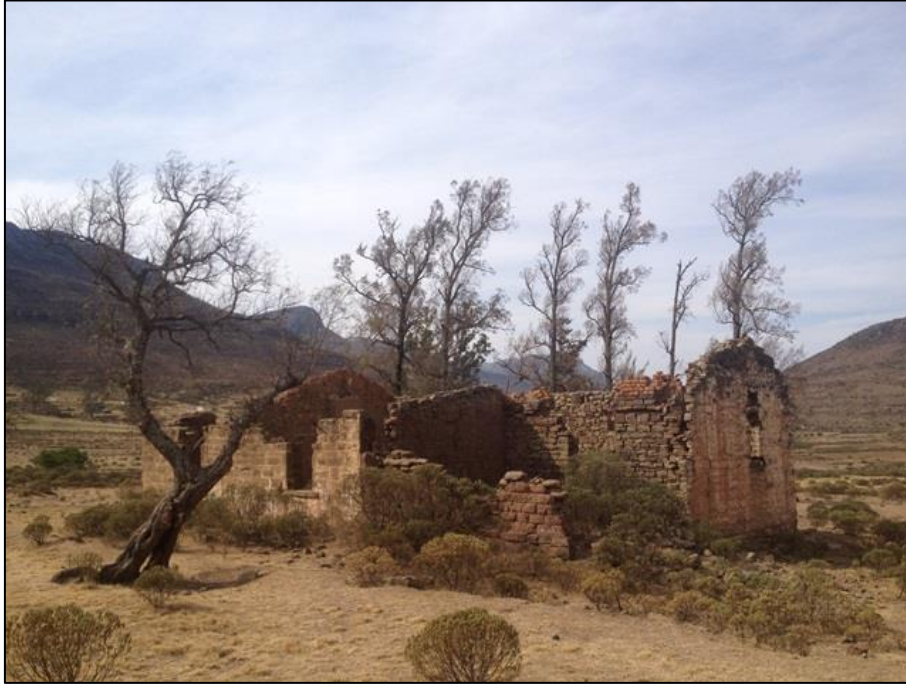
Figure 4-3: The dilapidated remains of a Historical Period farm house at Site LKH01.
