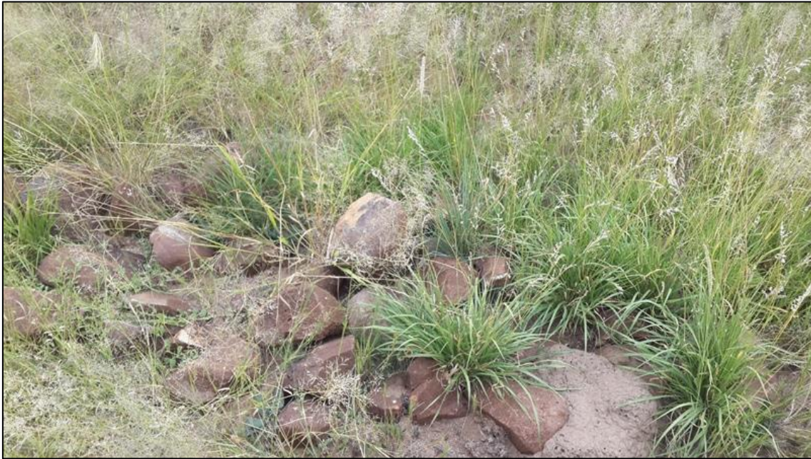
Figure 4-4: View of an overgrown and collapsed stone wall section at Site AGES-BW728-IA01.
