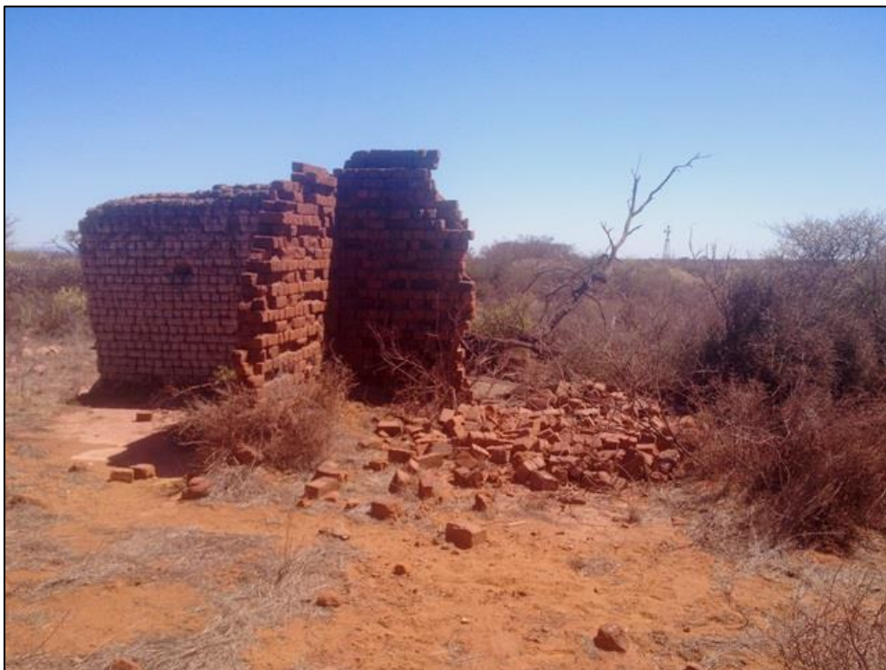
Figure 4-7: The dilapidated mud brick walls of the Woon farmhouse.
