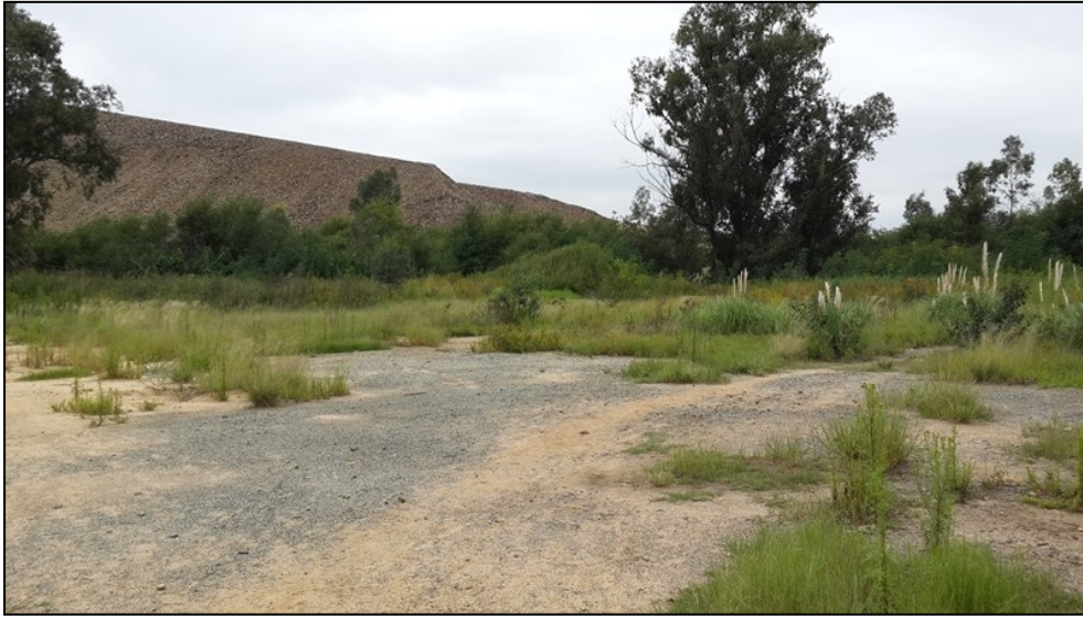
Figure 3-3: View of a cleared area in the project footprint where warehouses were demolished. Note old mine dumps in the distance.
