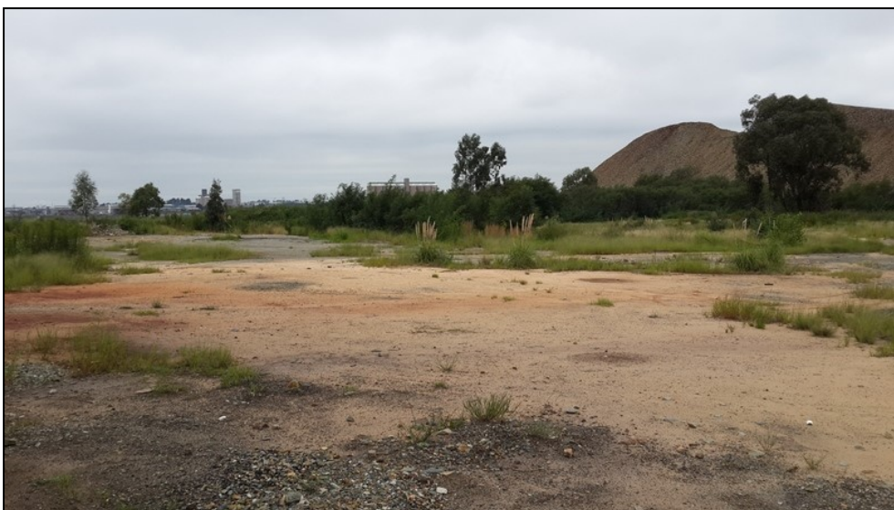
Figure 3-2: View of a cleared area in the project footprint where warehouses were demolished.
