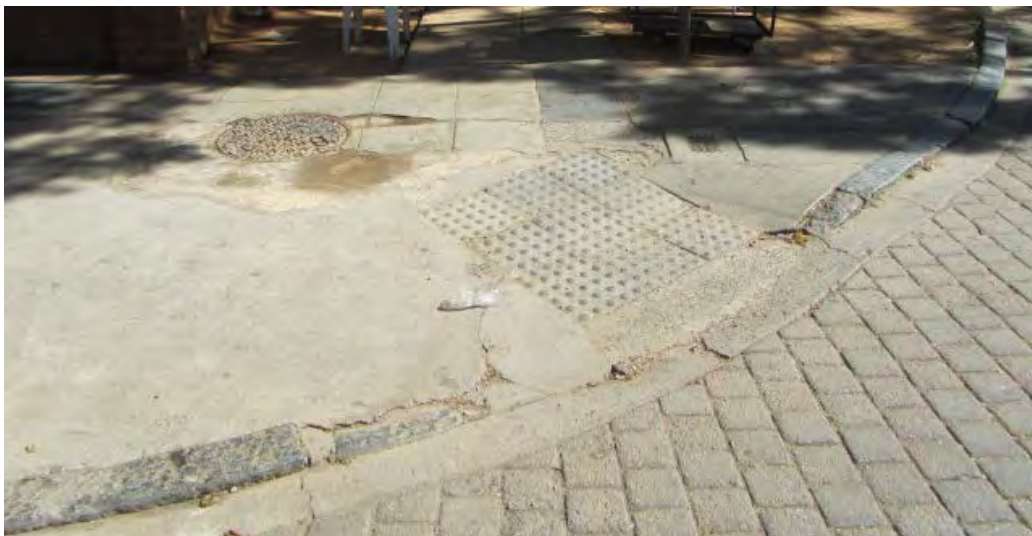
Fig. 148 Wheelchair access where the historical granite kerbing typically has been removed to adjust levels. (Photograph SM Miller 2012)
