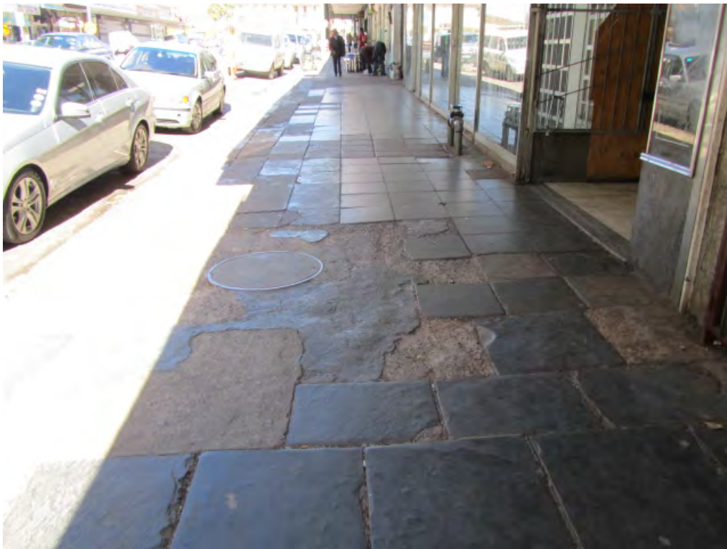
Fig. 164 Termination of the slate flagstone paving in the central western side of Block 10. Note the general condition of the modern paving. (Photograph SM Miller 2012)
