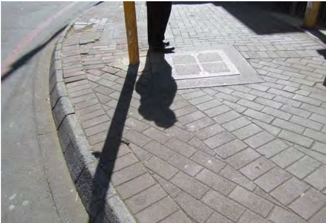
Fig. 96 Modern paving and kerbing possibly associated with the original broadening of Nana Sita Street. (Photograph SM Miller 2012)
