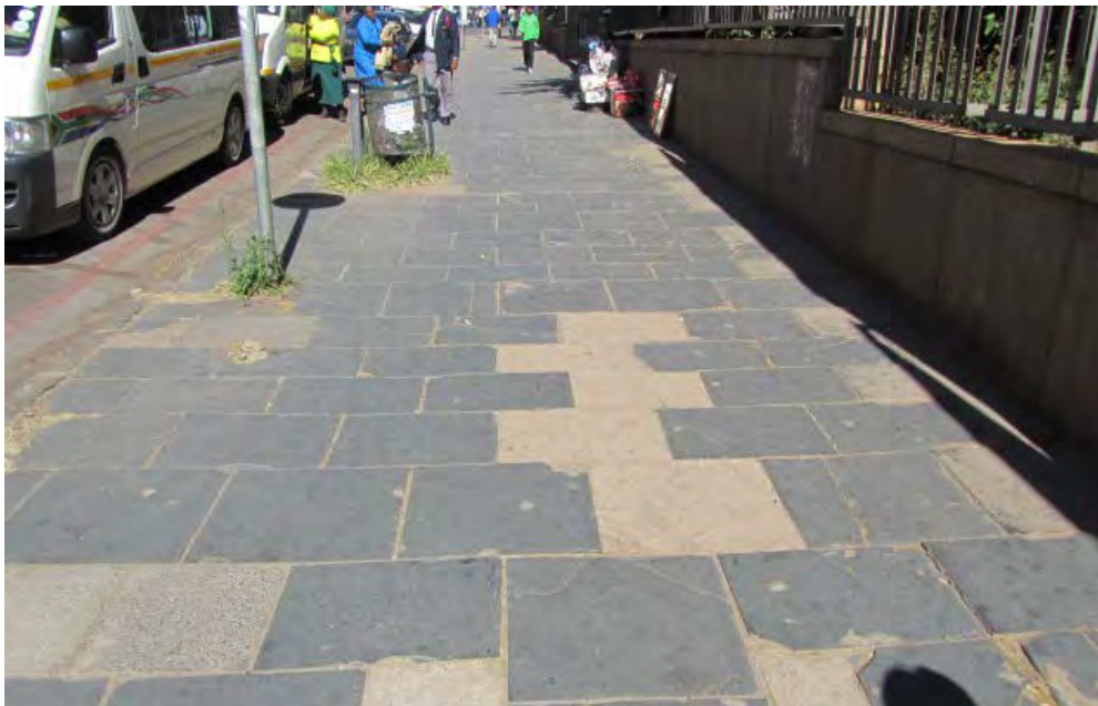
Fig. 152 In the south-western half of Block 9 most of the original slate flagstone paving remains. As elsewhere in the study area the paving is in a poor state of repair. Note variation in pattern of different types of flagstones. (Photograph SM Miller 2012)
