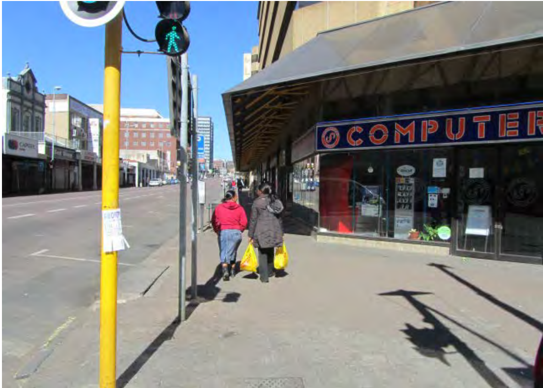
Fig. 77 North-western corner of Block 5. Culverts of various lengths and variable locations intrude on historical granite kerb stones, often close to street corners. (Photograph SM Miller 2012)
