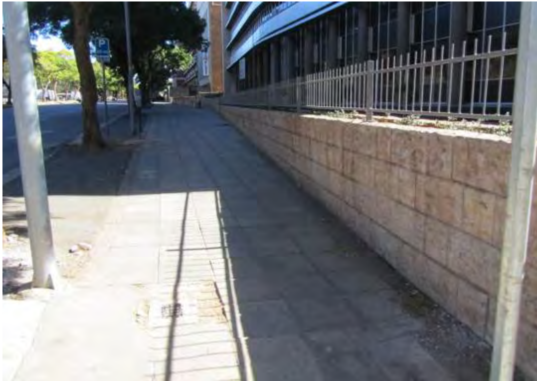
Fig. 113 Note condition of the paving along Visagie Street from Paul Kruger Street. (Photograph SM Miller 2012)
