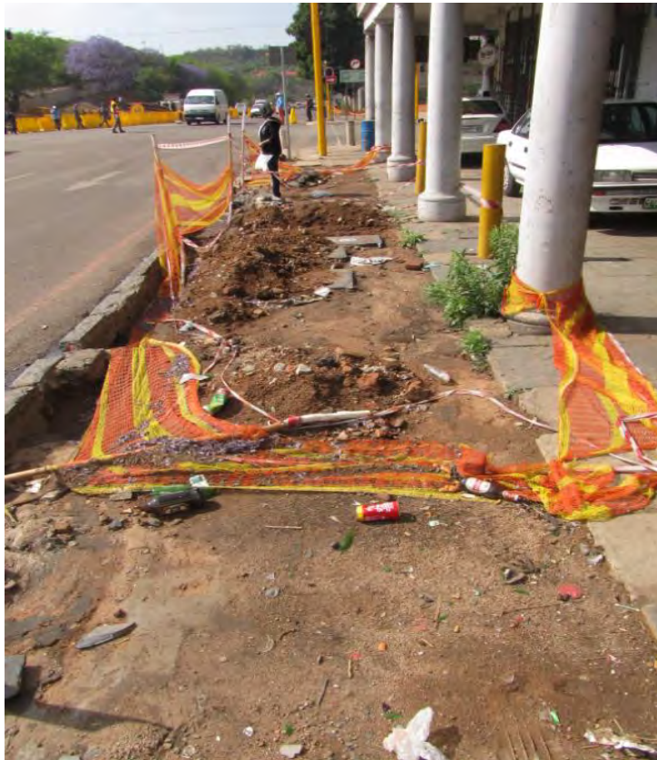
Fig. 20 Above is the historical slate flagstone sidewalk in front of protected building after an exploration for services. Compare to Figure 4. (Photograph SM Miller 2013)
