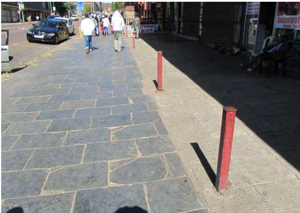
Fig. 108 Another section of slate flagstone paving on the western side of Block 7. Here only rectangular units were used. (Photograph SM Miller 2012)
