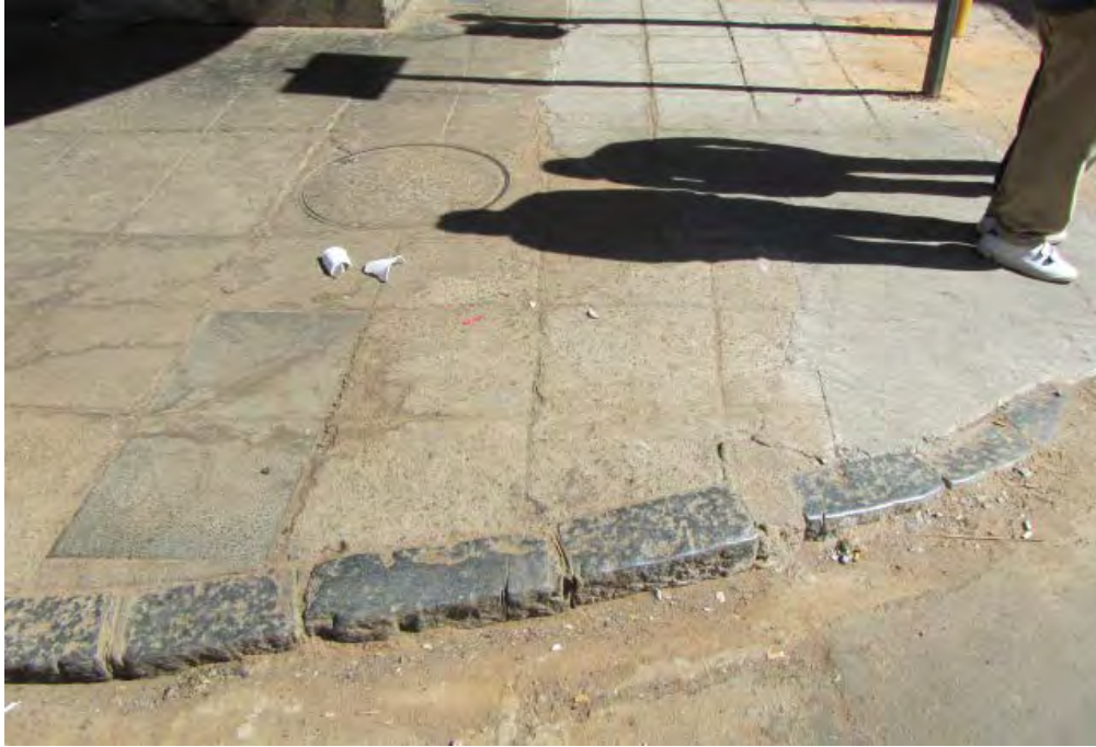
Fig. 90 A range of paving material and the granite kerbing. Note the use of short sections to create a corner radius. (Photograph SM Miller 2012)
