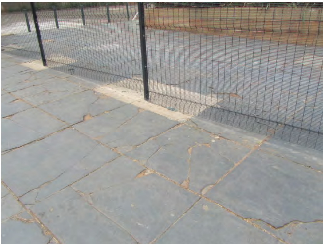
Fig. 136 The above image captures the current state of preservation of the slate flagstones in front of the Old Town Hall. It is estimated that no more than 10 to 20 percent of the large format (three feet square) flagstones are still intact. (Photograph SM Miller 2013)
