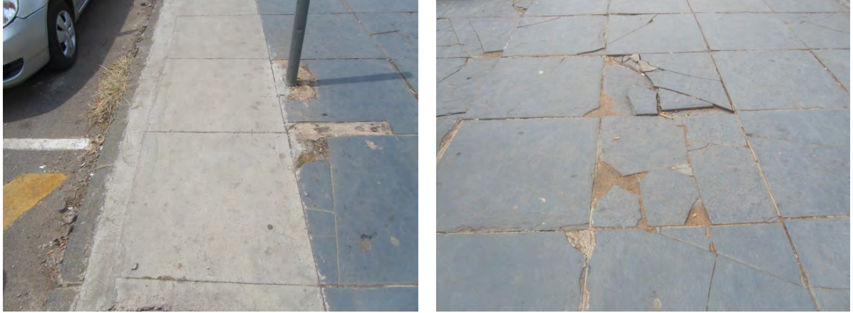
Figs 132 and 133 Both the above images illustrate how the placement of services and damage to flagstones over the past century have left the surface in a poor state of repair. (Photograph SM Miller 2013)
