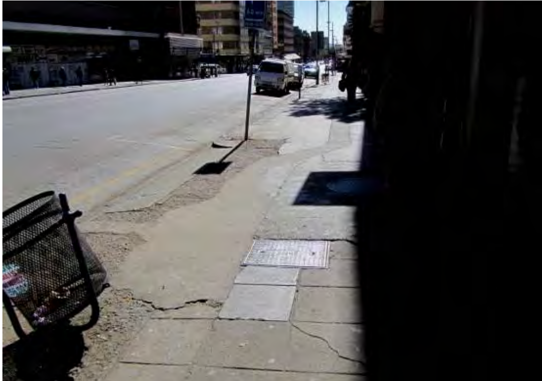
Fig. 97 A variety of paving material suggesting a perceived lack of standards for the construction of Tshwane sidewalks. Also note the vehicular access area. (Photograph SM Miller 2012)
