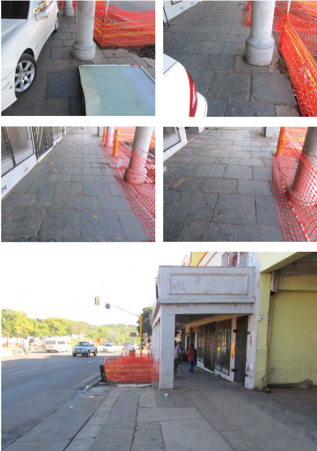
Figs 15 to 19 Above can be seen historical slate flagstones on the sidewalk in front of a protected building in Block 1 on the eastern side of Paul Kruger Street.
