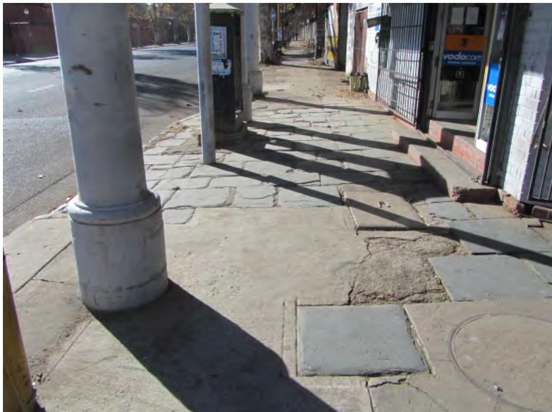
Fig. 8 Historical slate flagstones, granite kerbing and pillars of sidewalk in front of protected building. (Photograph SM Miller 2012)
