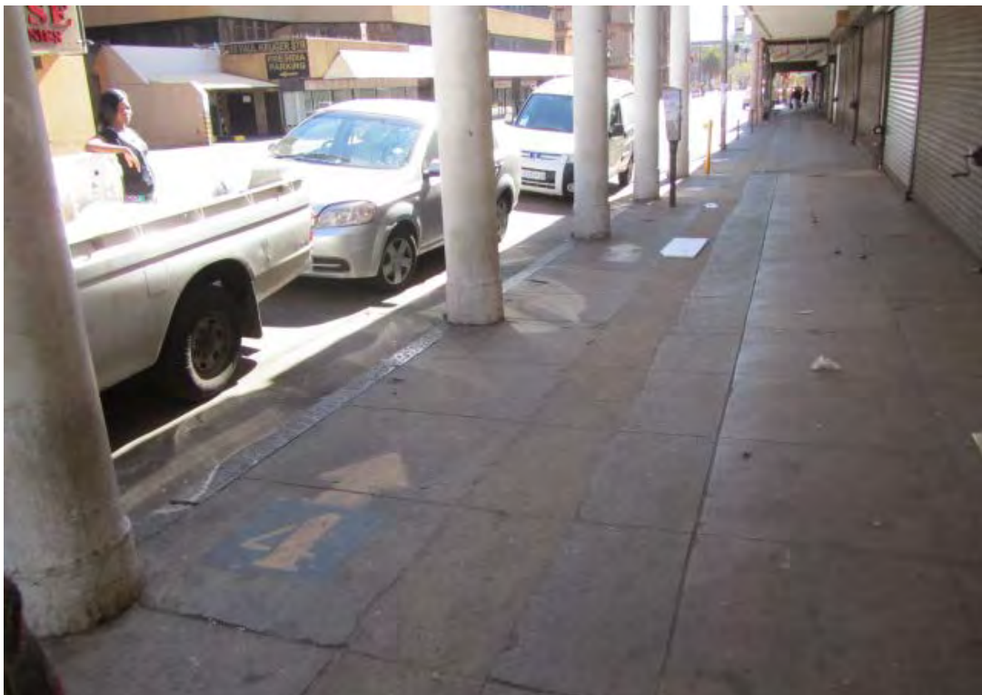
Fig. 83 Granite kerbing on the central eastern side of Block 5. Fracturing of the granite kerbing at column bases probably explains the discontinuation of granite kerbing elsewhere along the street. (Photograph SM Miller 2012)
