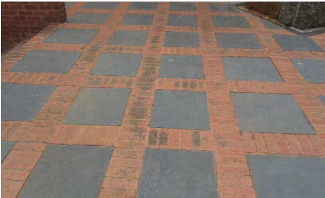
Fig. 128 With the extension of the Museum Building some years ago the original paving was removed and replaced. This is an example where some form of the historical slate flagstone paving has been retained. The poor preservation of the flagstones, which can be seen in front of the Old Town Hall, probably required a combination of original and new paving. Although attractive and well designed, it should be the last option where original paving exists. (Photograph SM Miller 2012)
