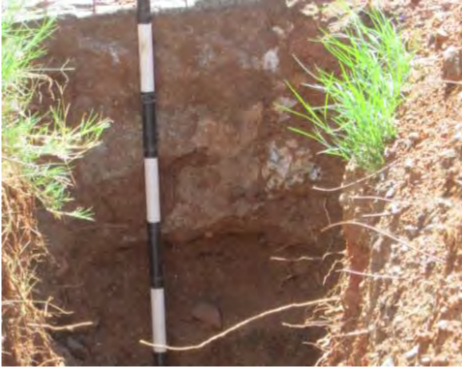
Fig. 60 The above photograph records the depth of the granite kerbing on the east side of Block 3, being around 350 mm (7 inches). This may vary as the kerb stones were handmade. (Photograph SM Miller 2013)
