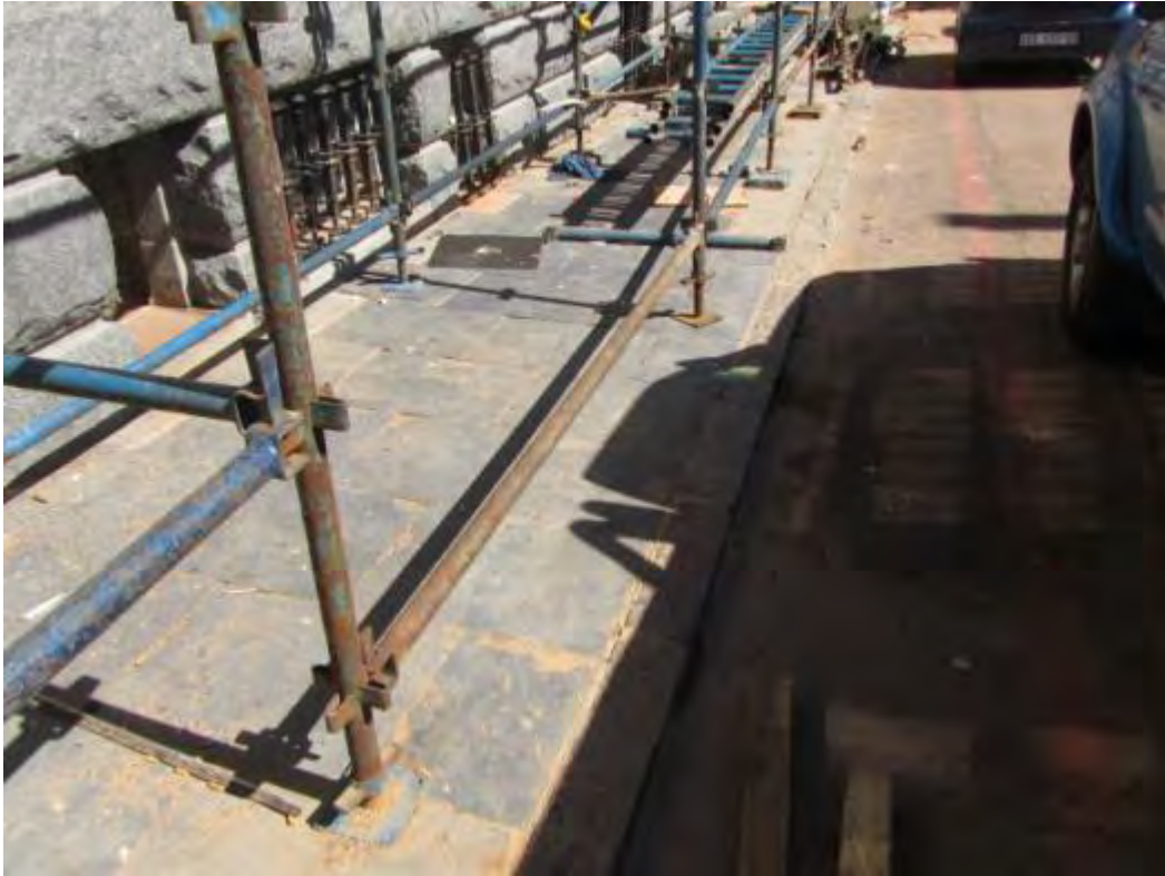
Fig. 38 Improper placement of scaffolding on historical slate paving. (Photograph SM Miller 2013)
