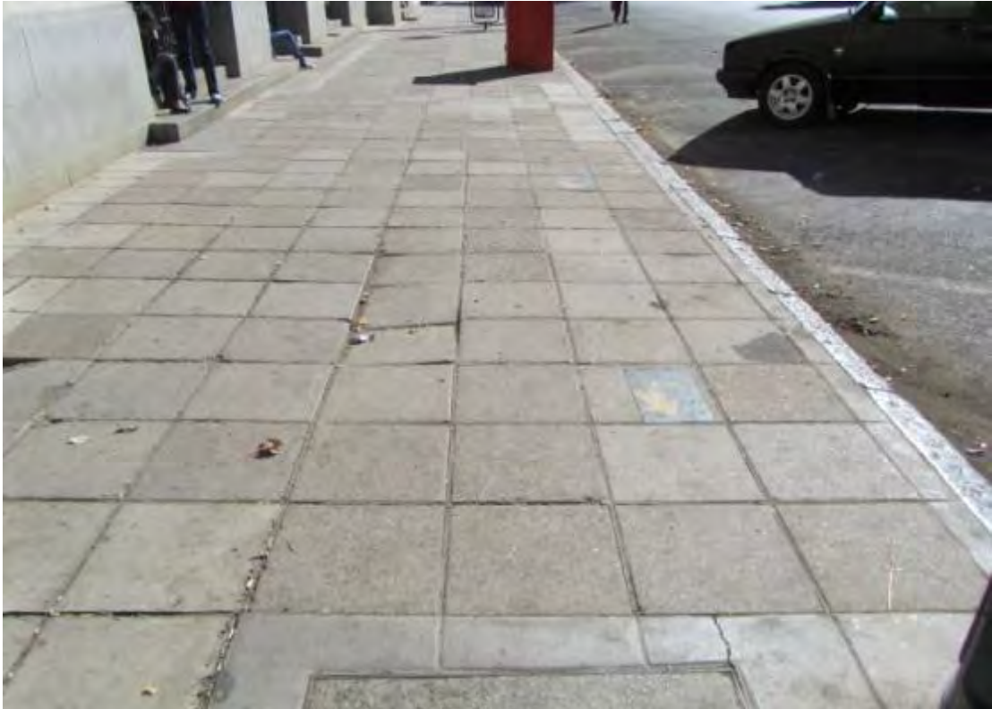
Fig. 31 Modern paving and historical granite kerbing along the western section of the Square. (Photograph SM Miller 2013)
