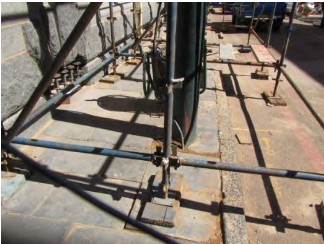
Fig. 35 Historical slate paving and historical granite kerbing along the south-western section of Block 2 under scaffolding for restoration on the Mutual Insurance Building. (Photograph SM Miller 2013)
