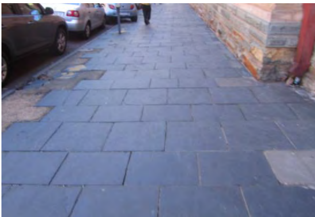
Fig. 23 Historical slate flagstone paving and historical granite kerbing along the north-eastern section of Block 1. It appears as if these flagstones may have been lifted, trimmed and re-laid in recent times. (Photograph SM Miller 2013)
