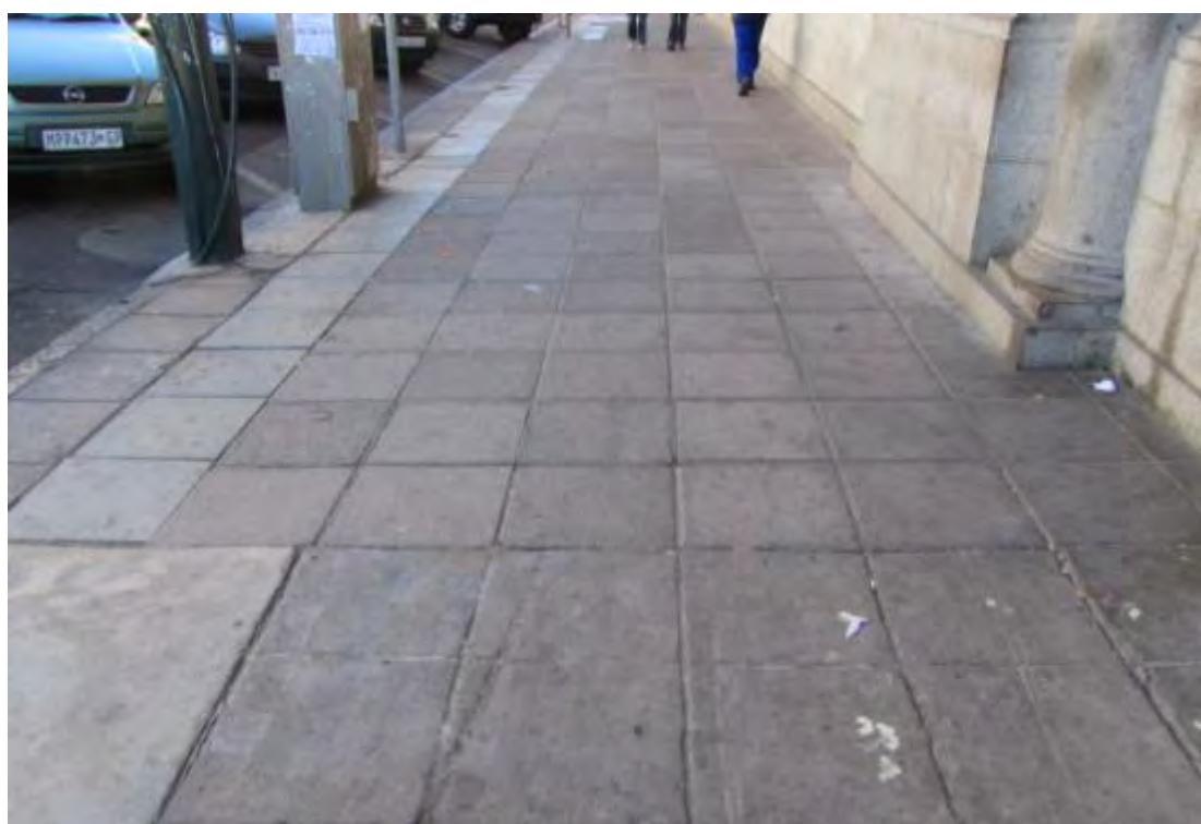
Fig. 31 Modern paving and historical granite kerbing along the western section of the Square. (Photograph SM Miller 2013)
