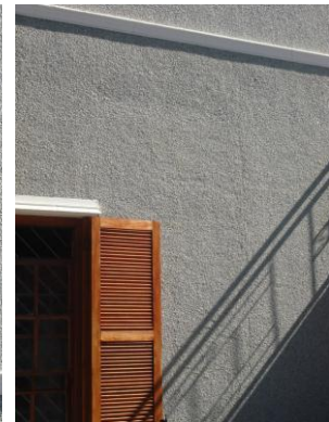
Evidence of old doorway
