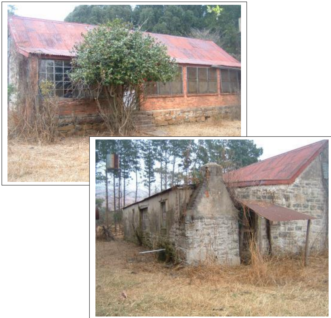
Figures 6 & 7- HH01 dates from AD1903 and viewed from the front (above) and back (below). The original house has been extended on both these.
