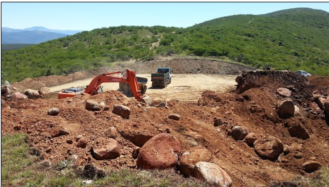
Figure 8: The Sandile Water Treatment Works Reservoir construction site at the time of the site inspection in January 2015, looking north.
