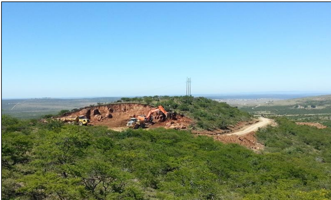
Figure 7: The Sandile Water Treatment Works Reservoir construction site at the time of the site inspection in January 2015, looking south.
