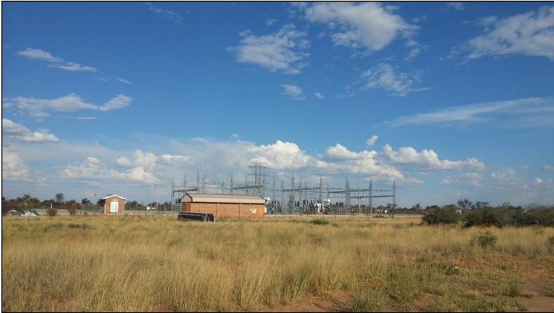
Figure 3-10: View of the Umtu Substation and the southern offset of Corridor 2.
