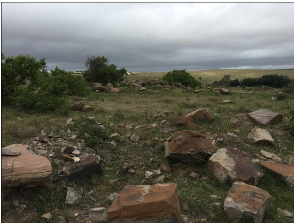
Figure 5-4: Scattered stones and dilapidated stone wall structures at site EXIGO-CWS-FT01.
